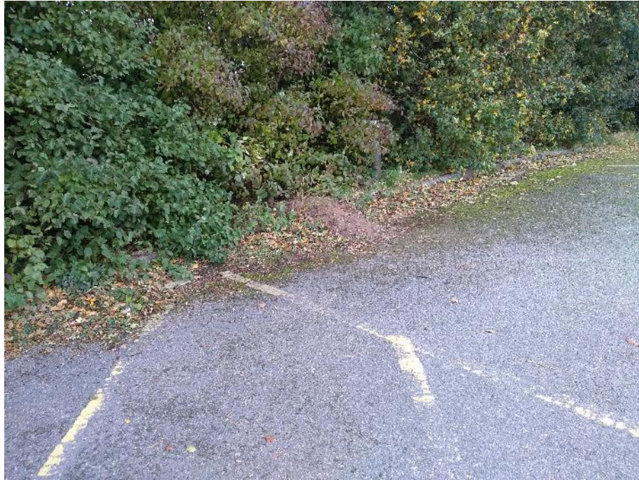
Figure 4: Image of dirt overflowing onto hardstanding due to sett digging in 2021
