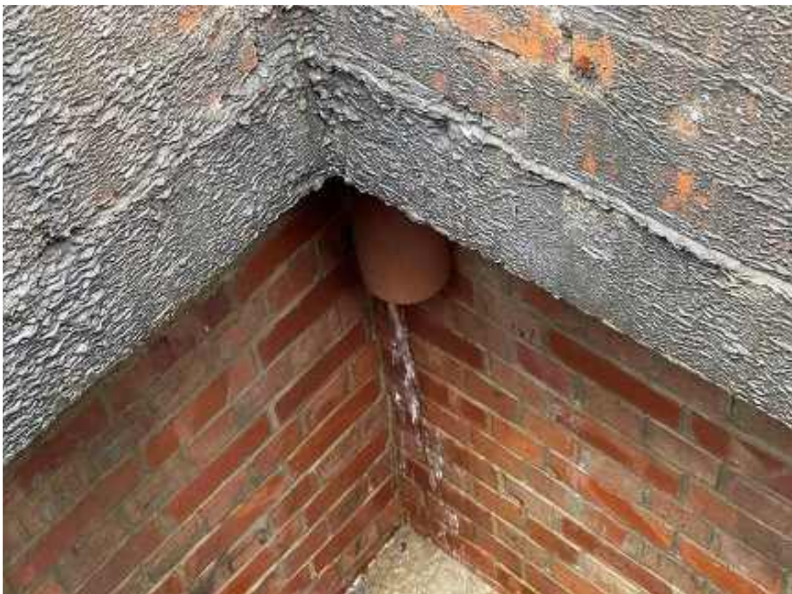
MH S8 (WATER CONTINUALLY RUNNING INTO MANHOLE)
