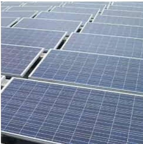
PV Panels: Rooftop Solar Panels
