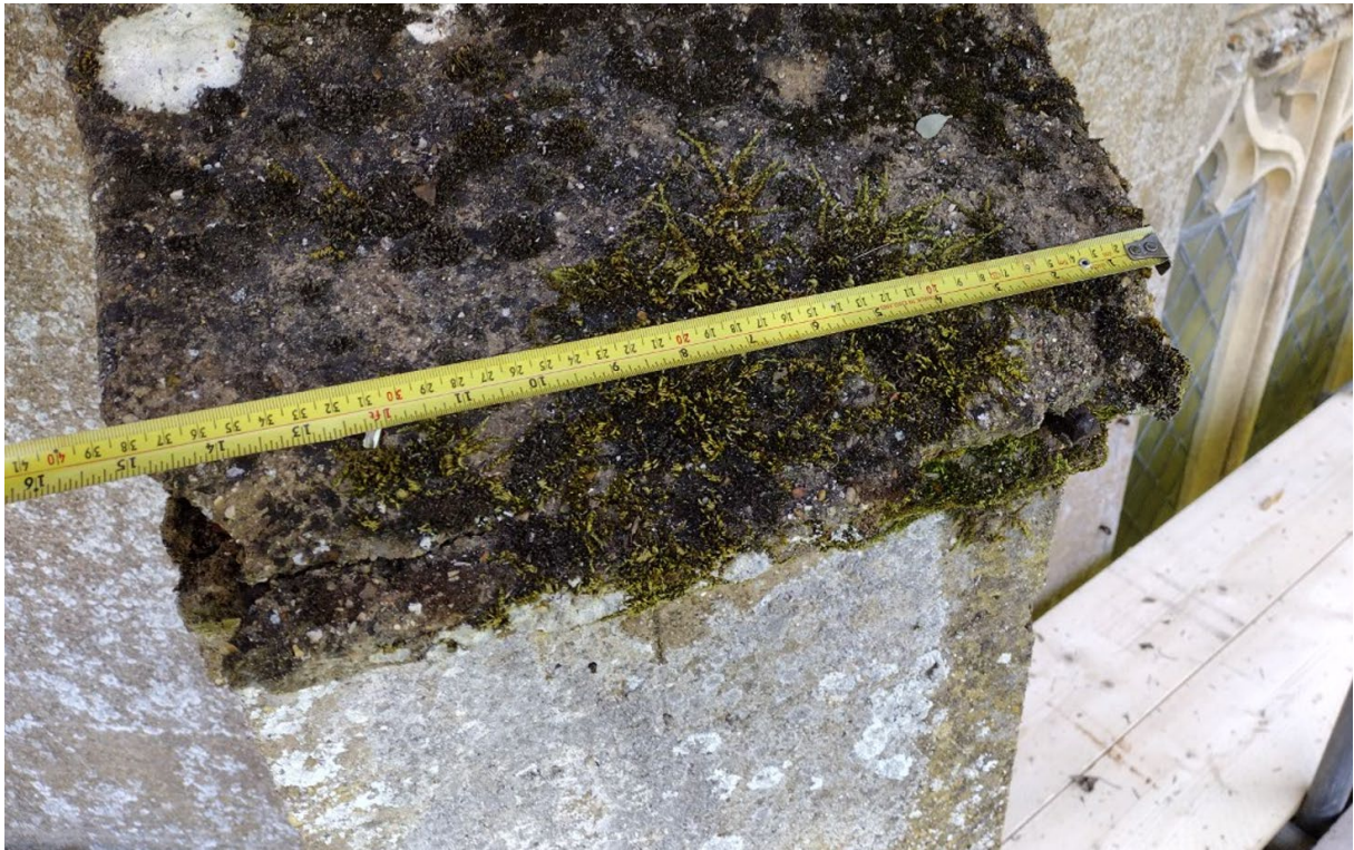
Fig 22: Buttress corbel to be cleaned of moss with local render repairs.
