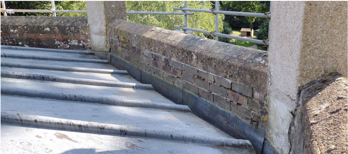
Fig 18: Areas of repointing required to inside face of parapet wall.
