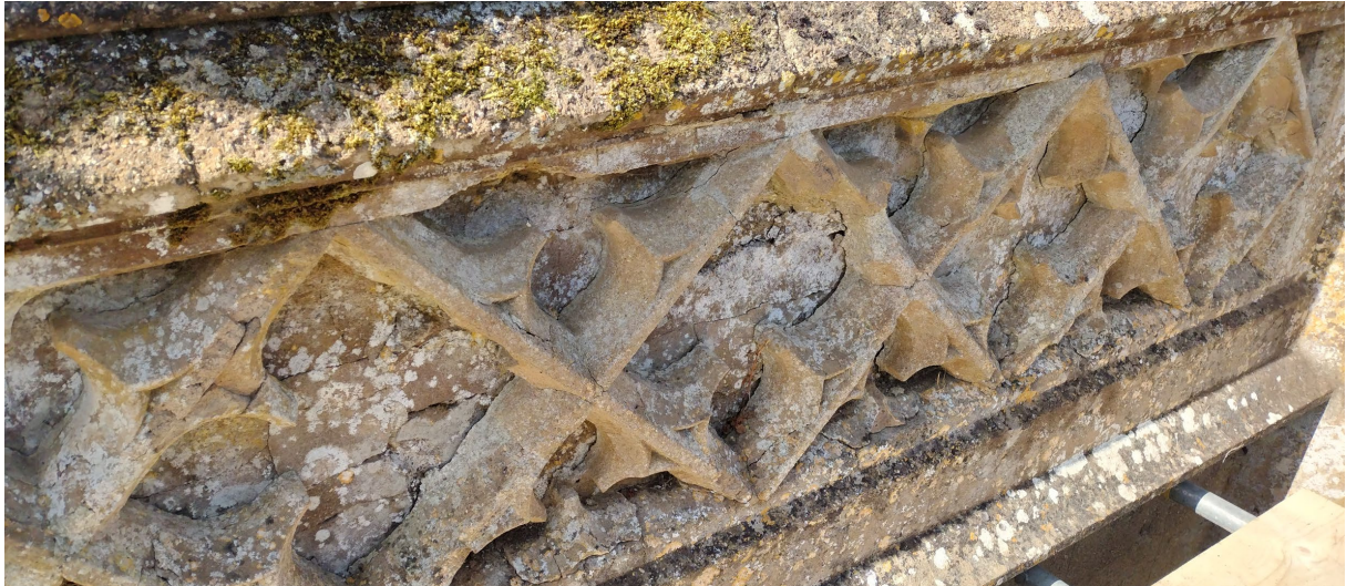
Fig 19: Areas of pointing required to stabilise the Quatrefoil, to avoid hazard of falling masonry.
