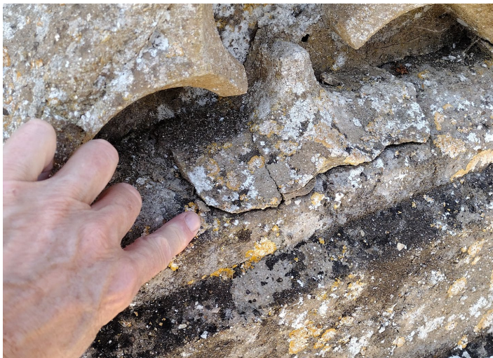
Fig 20: Areas of stabilisation of the Quatrefoil, to avoid hazard of falling masonry.
