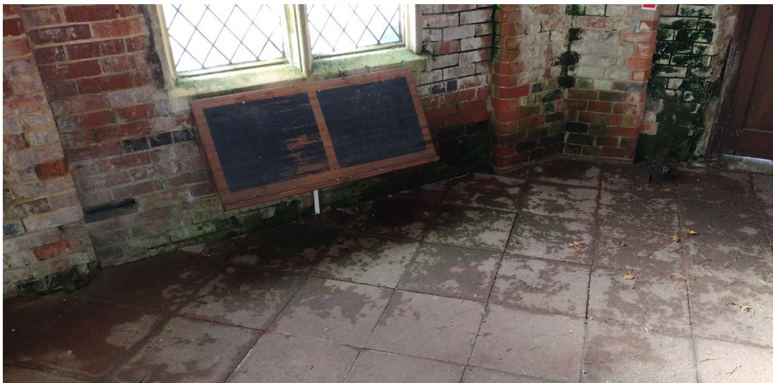
Fig 7: Image showing damp floor.
