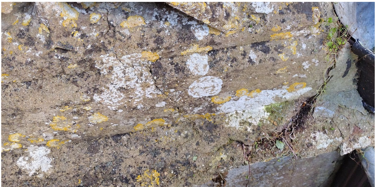
Fig 21: Identified areas of stabilisation to the flounced ledge.
