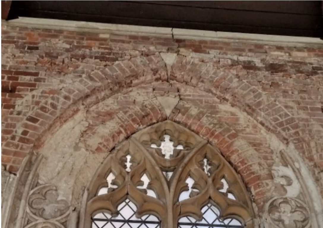
Fig 10: Image showing masonry cracks above arch windows
