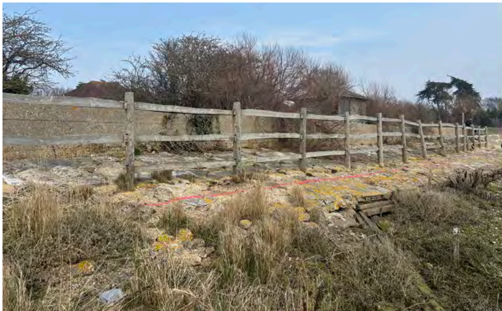
Figure 9. View of concrete skirt showing edge south of wooden fence in poorer condition (taken March, 2025).
