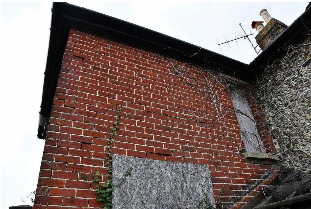
PLATE 28: Close-up on (27) above showing stepped diagonal cracking running up from corner above window level – possible evidence of previous repairs?
