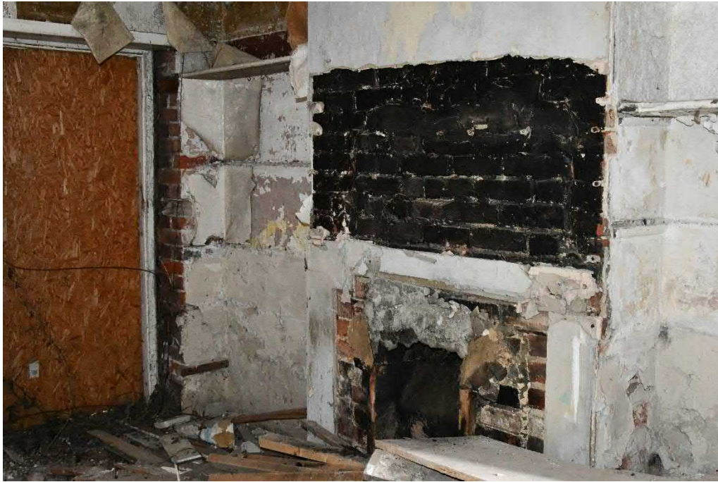
PLATE 41: Damage from removal (theft?) of fireplace
