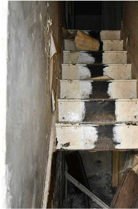
PLATE 39: Lower part of staircase removed preventing access to first floor
