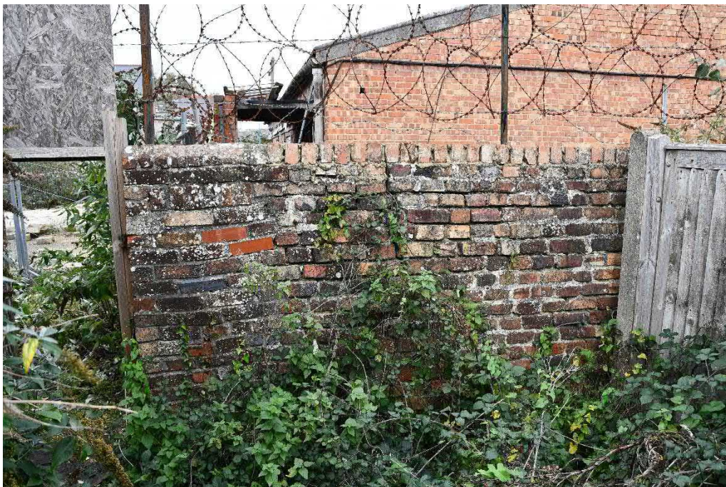
PLATE 36: Boundary wall on north side of site to east of house – note distortion to line of wall and loss of pointing
