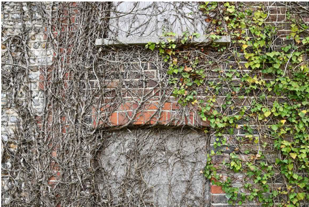
PLATE 10: Cracking to/above brick arch lintel to western ground floor window in (1) above
