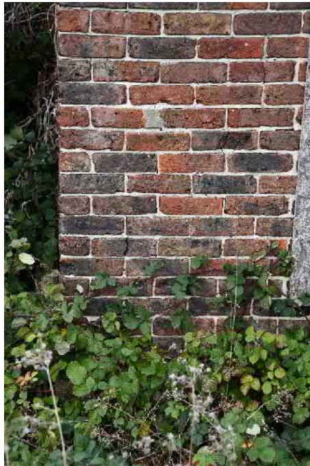
PLATE 18: Low level cracking between corner of wall and window reveal in (15) above
