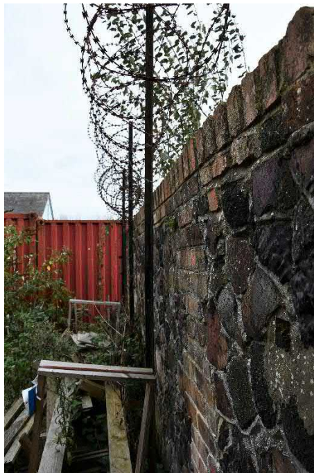
PLATE 38: View along north side of boundary wall in (36) above looking east – note slight outward lean to wall
