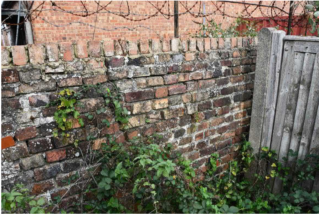
PLATE 37: Close-up on damage to wall in (36) above showing diagonal cracking to wall – note timber fence to substation to right of view
