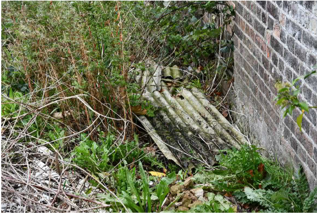
PLATE 11: Corrugated sheeting, possibly asbestos cement, on ground in front of western end of north elevation
