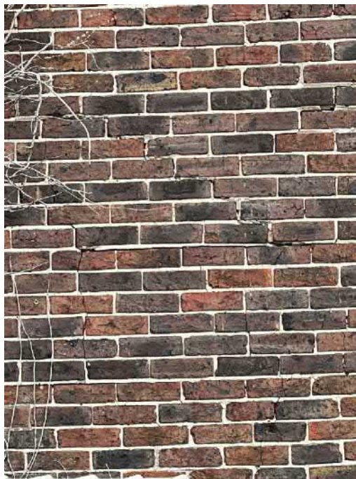
PLATE 14: Stepped diagonal and vertical cracking to gable wall parallel to corner at mid height immediately below view in (13) above
