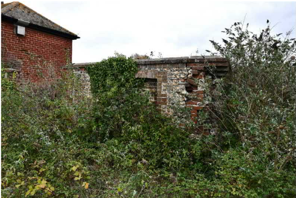
PLATE 22: Garden wall, possibly remnant building, running south from south-west corner of rear "extension – note cracking to corner of wall
