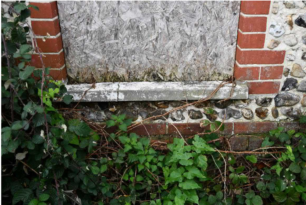
PLATE 35: Cracking to cill of ground floor window in (33) above
