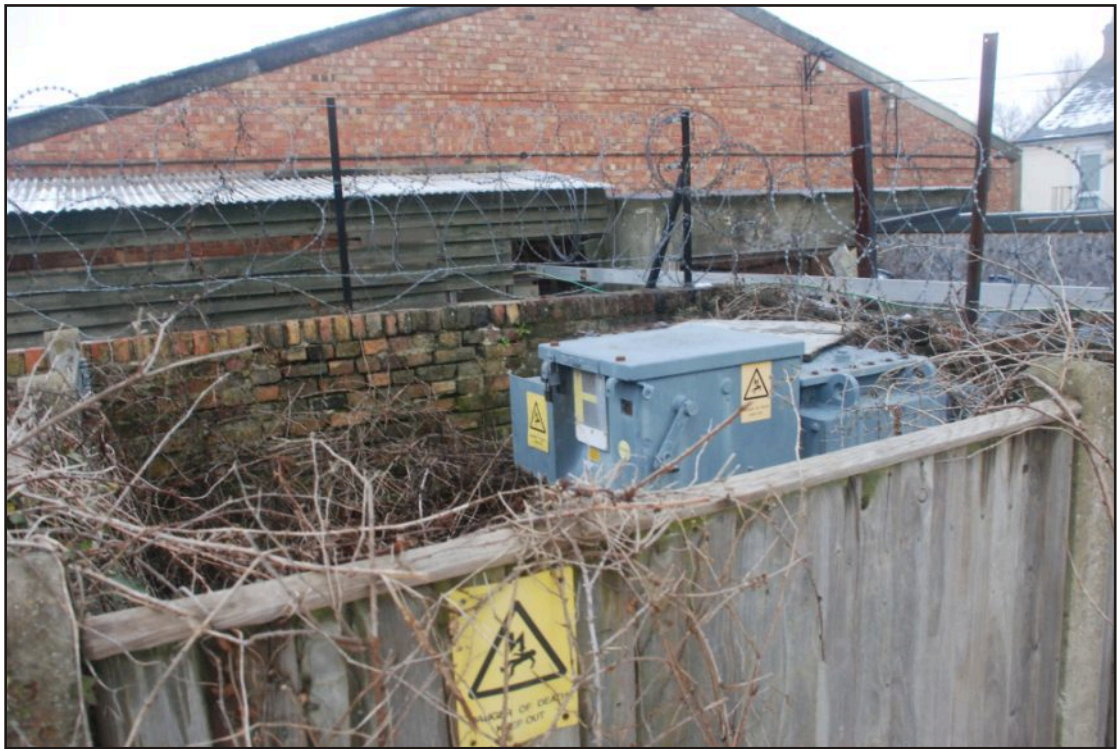
Plate 14. Second sub-station compound in north-eastern corner of site.
