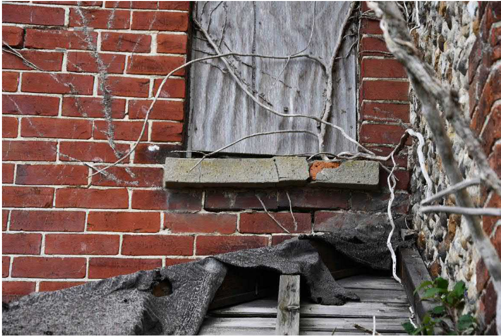
PLATE 31: Cracking to/beneath first floor window cill and slight "kick-out" in (30) above
