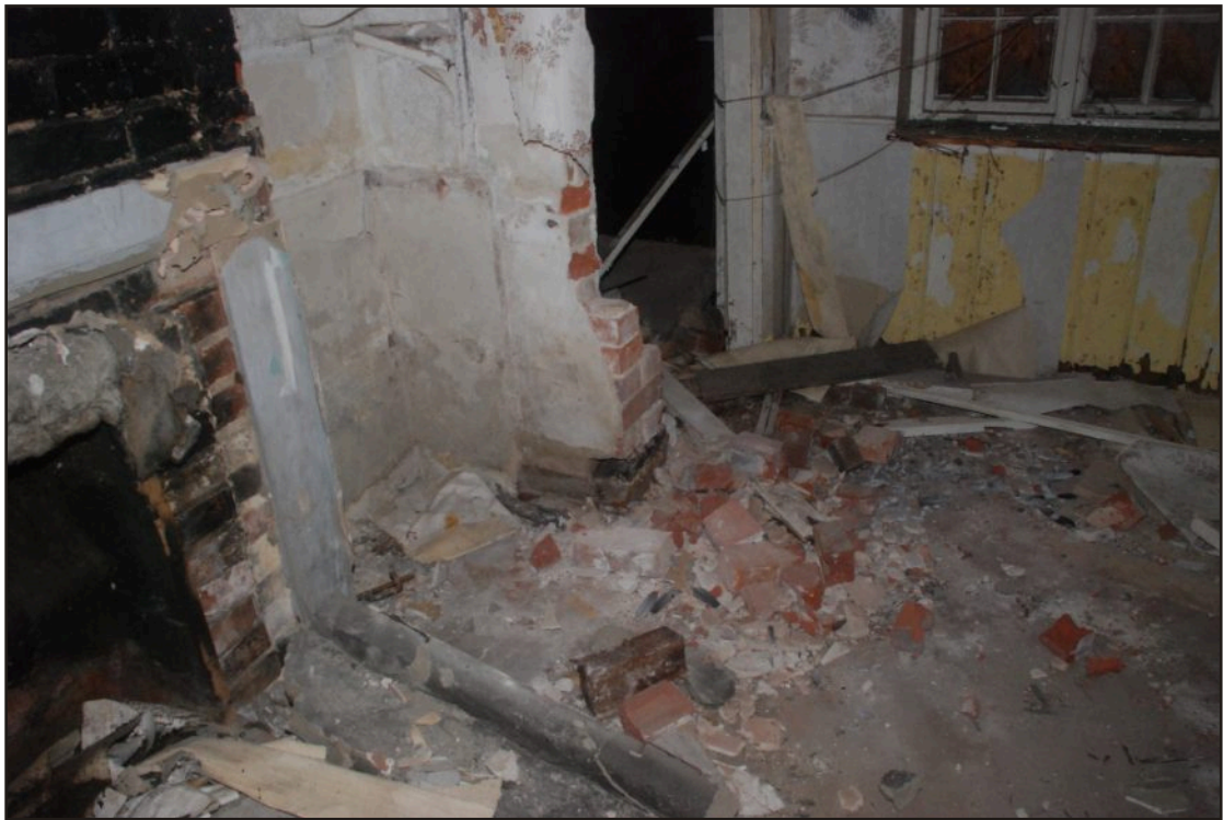
Plate 24. Further view on room in (23) above showing damage caused by removal of fireplace.
