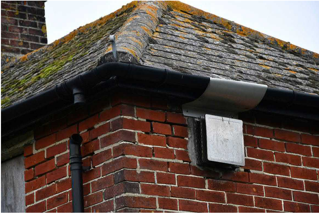
PLATE 21: Close-up on (20) above showing loss of pointing between window reveal and corner at eaves level and around vent
