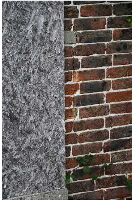
PLATE 17: Vertical crack parallel to window reveal in (15) above
