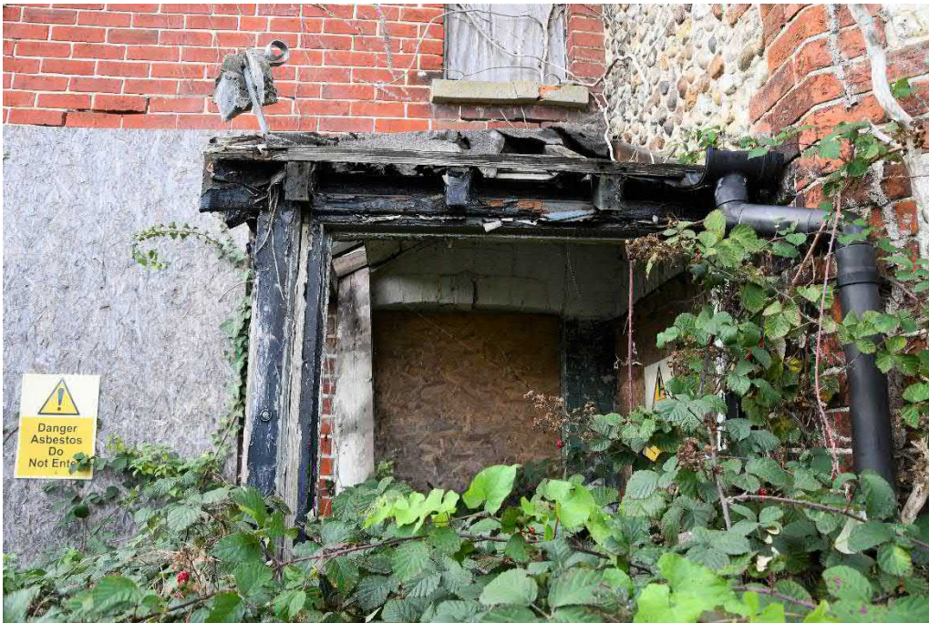
PLATE 32: Cracking to brick arch lintel over door in (30) above
