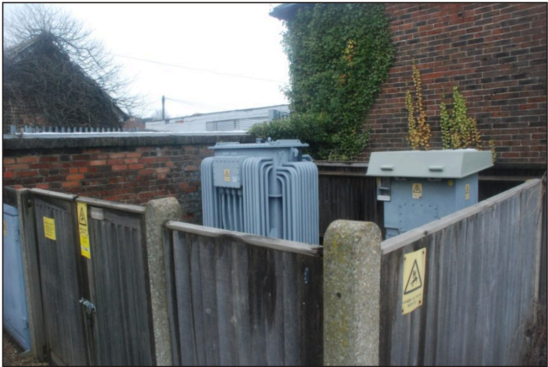
Plate 10. Close-up on sub-station in (9) above.
