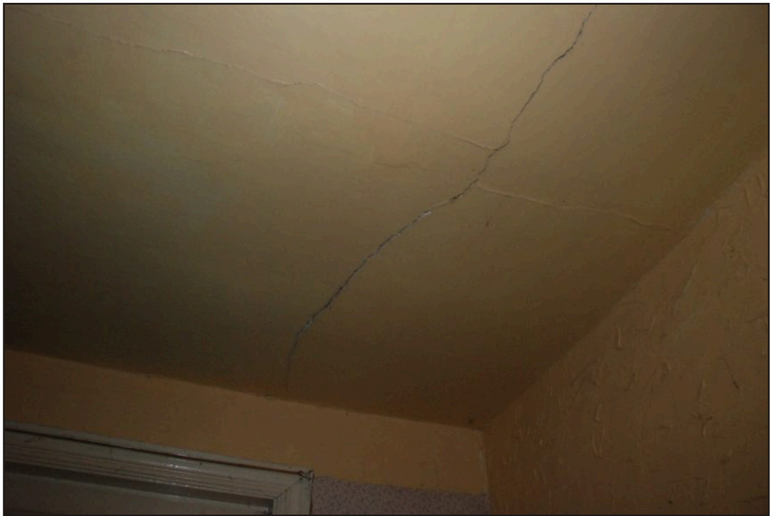
Plate 32. Ceiling cracking at first floor level.
