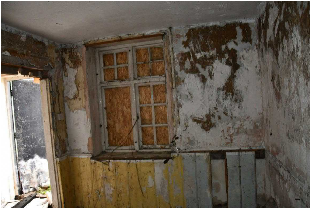
PLATE 42: Evidence of water damage to walls generally to ground floor
