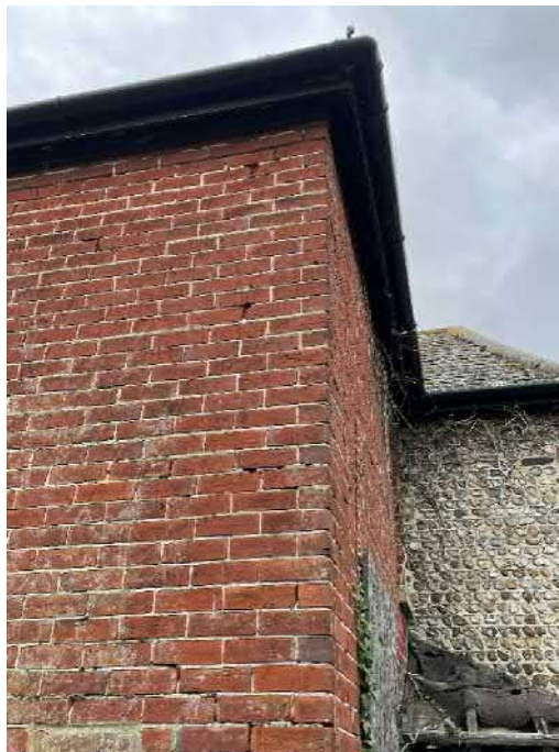
PLATE 24: Close-up on (23) above showing stepped diagonal cracking between first floor and eaves level
