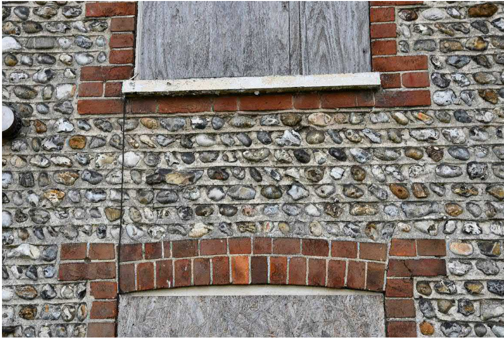
PLATE 9: Vertical cracking above both ends of brick arch lintel to eastern ground floor window in (8) above
