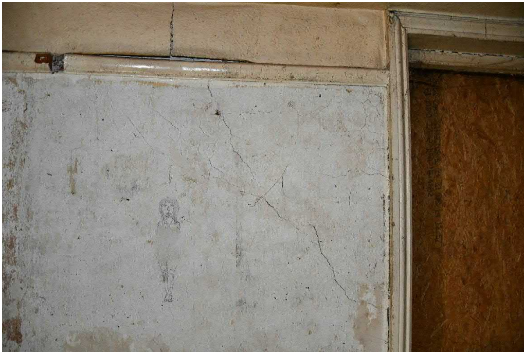
PLATE 46: Close-up on (45) above – note diagonal cracking to side of window reveal
