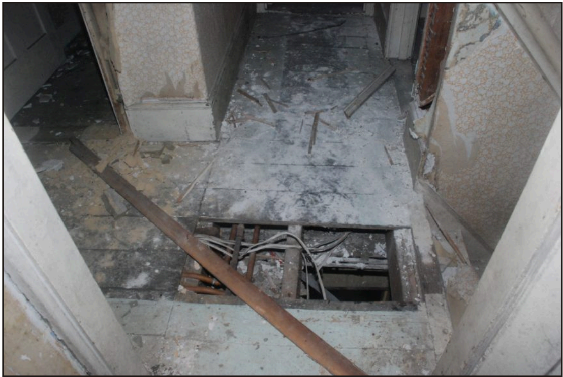
Plate 27. Missing floor boards at top of stairs to first floor.
