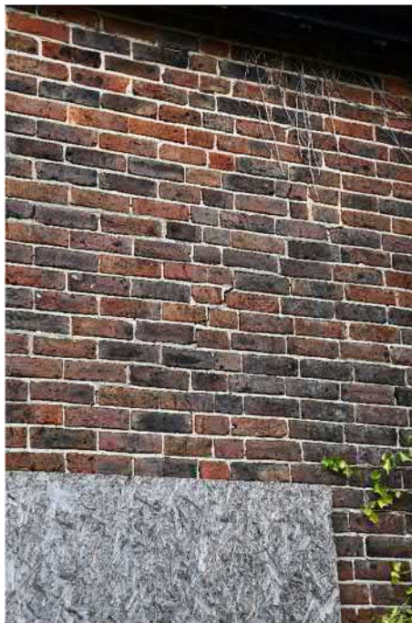
PLATE 16: Vertical crack from centre line of window up to eaves in (15) above
