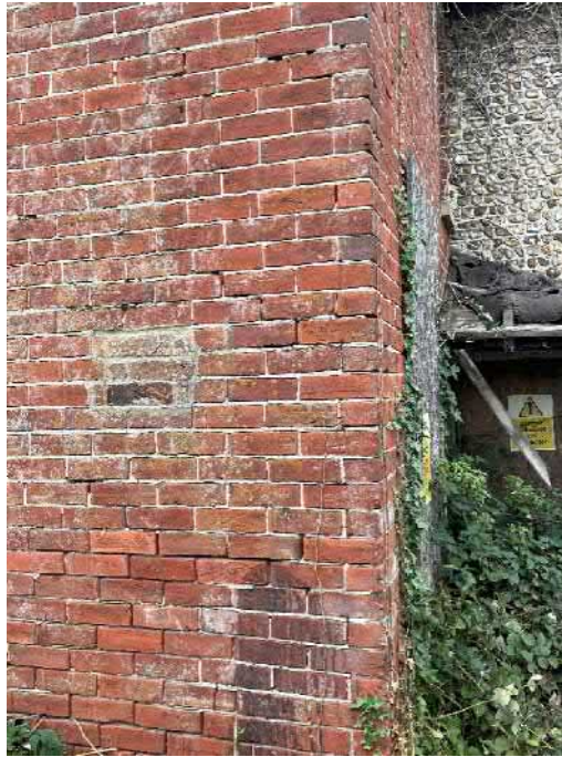
PLATE 25: Further view on (23) above showing loss of pointing at low level with stepped diagonal cracking above
