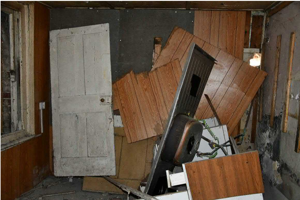
PLATE 44: Extensive damage/theft/vandalism within property
