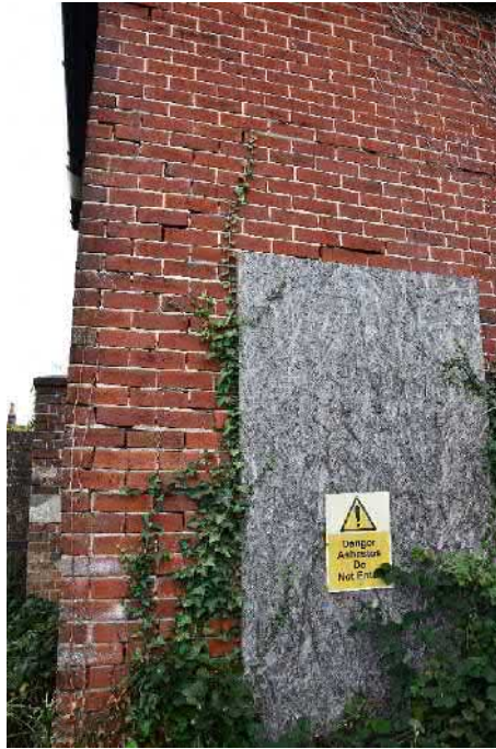
PLATE 29: Cracking and distortion of wall between window reveal and corner in (27) above – possible evidence of settlement?
