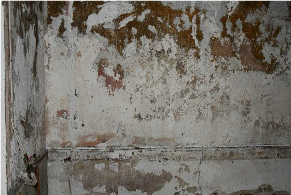
PLATE 43: View on eastern wall of house showing two parallel vertical cracks to full height of ground floor – possible infilled opening?
