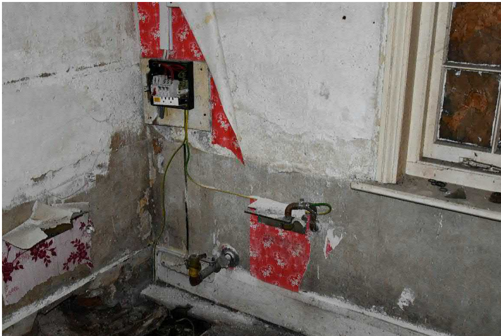
PLATE 48: Close-up on (47) above – gas and electricity meters removed
