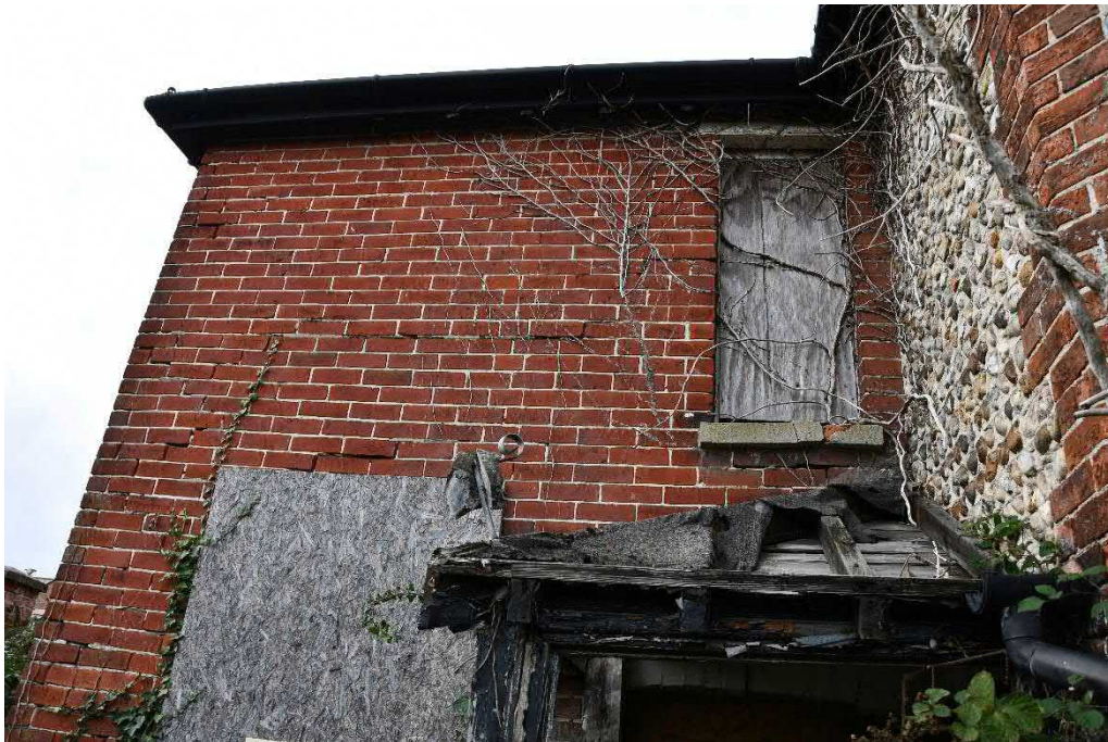
PLATE 30: Further view of (27) above - note cracking above lintel to ground floor window and slight bowing of wall
