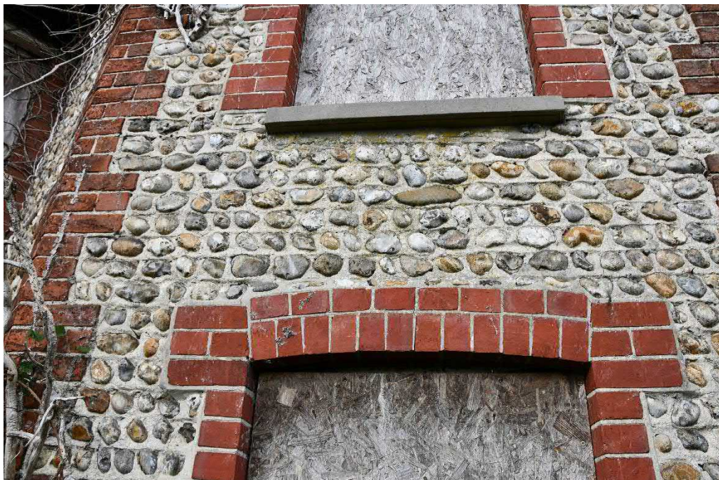
PLATE 34: Vertical cracking above both ends of brick arch lintel to eastern ground floor window in (33) above
