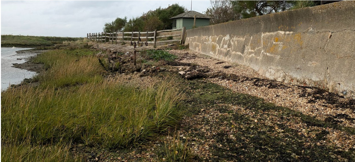
Poor condition of sea defence wall adjacent Number 8 Harbourside (Oct 2024)
