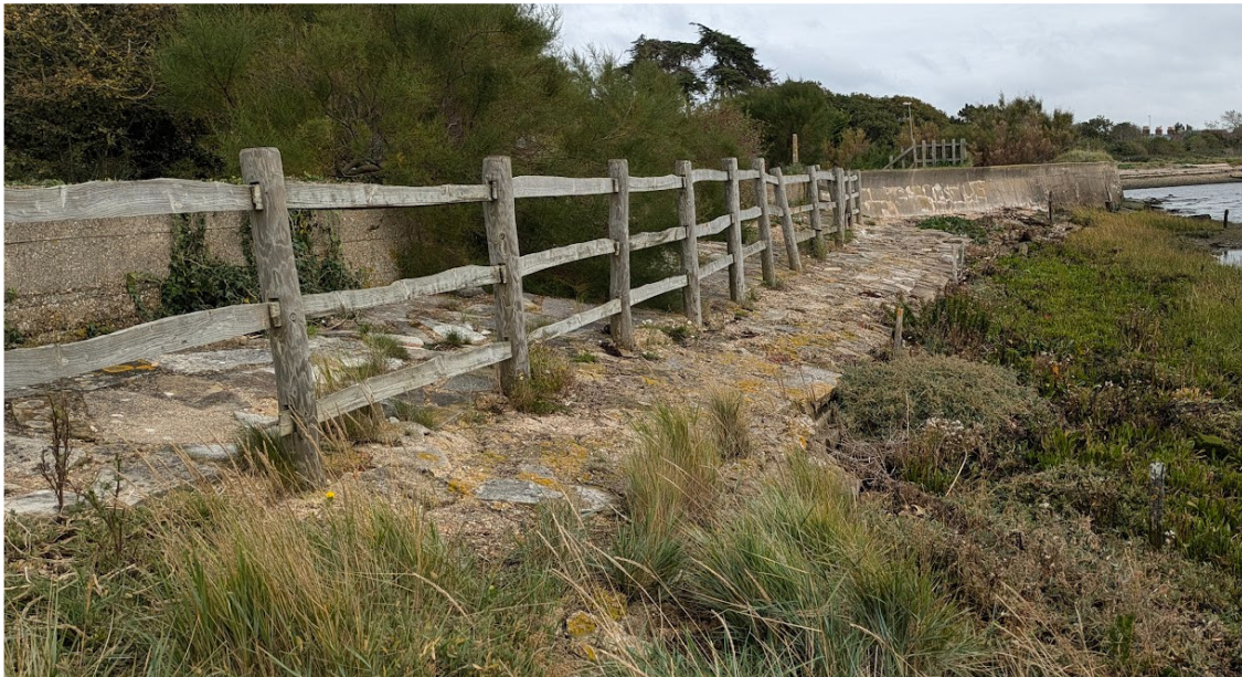
Poor condition of sea defence wall adjacent Number 9 Harbourside (Oct 2024)
