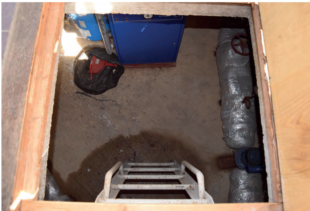
Plate 460: Technical room under ground floor.
