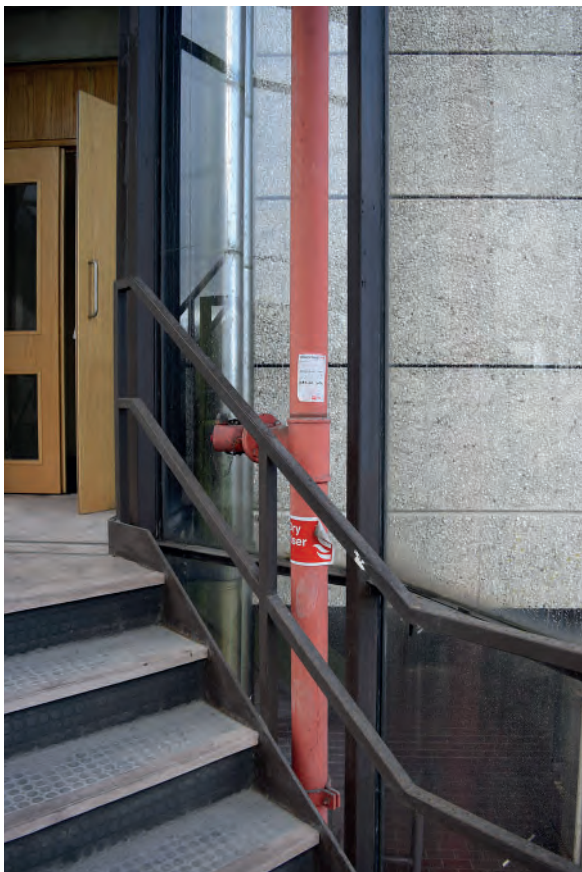
Plate 464: First Floor, hydrant, looking west.
