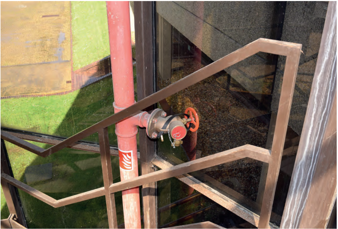
Plate 483: First Floor, hydrant, looking north.
