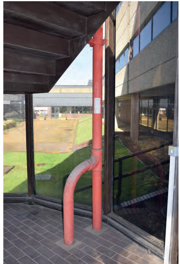
Plate 477: Ground Floor, hydrant, looking north.
