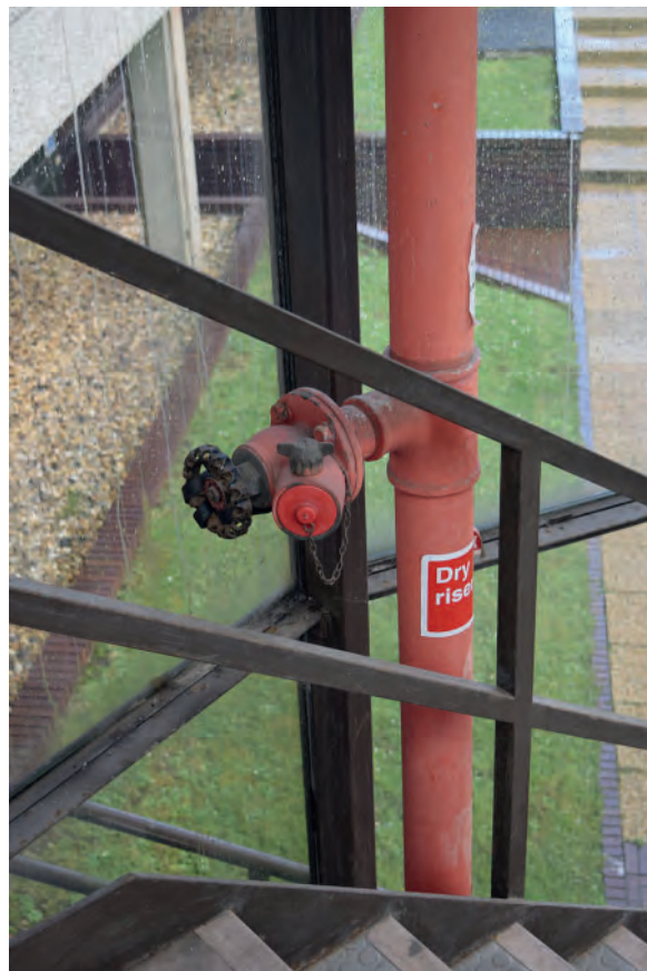
Plate 465: First Floor, hydrant, looking north.
