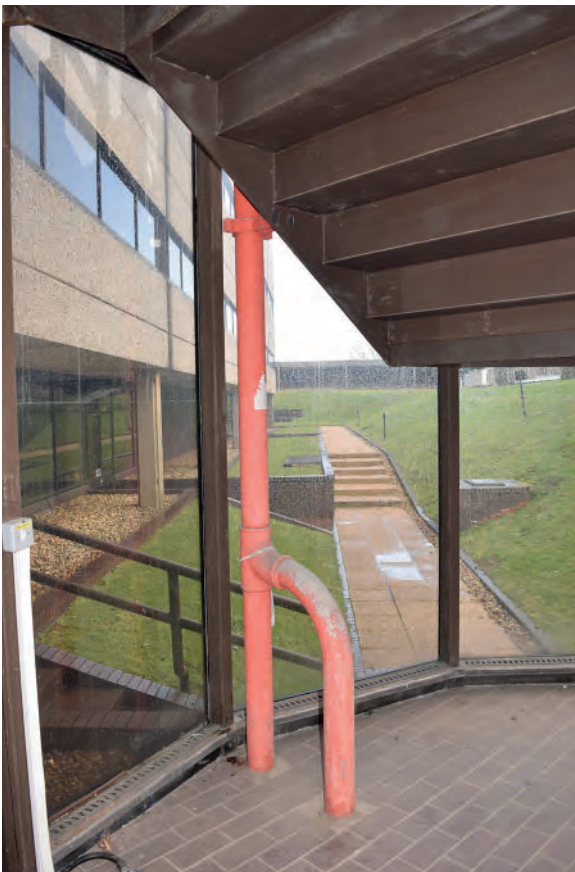
Plate 462: Ground Floor, hydrant, looking north.
