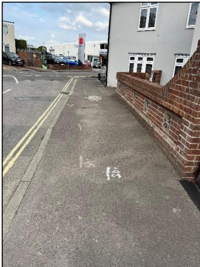
Photograph 2: Palk Road southern footway
