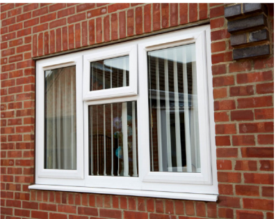
uPVC Double Glazed casement windows
