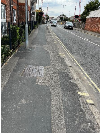
Photograph 12: West Street footway to Bedhampton rail station
