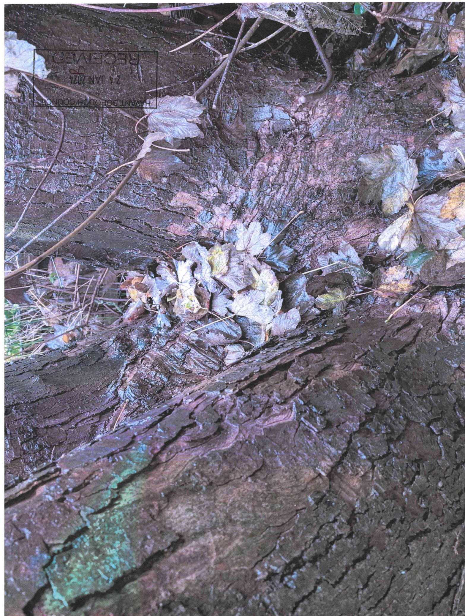
BASE OF 3 SYCAMOLES, ST THOMAS' CHURCH BEDHAMPTON
