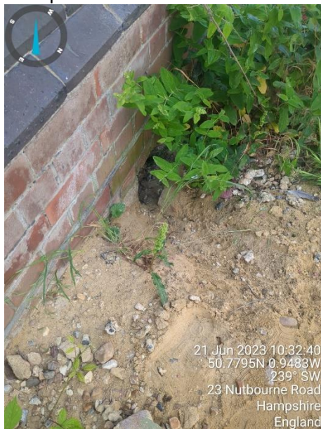
Photograph 19: View of a mammal burrow underneath the foundations on the northern elevation of the building.
