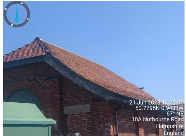
Photograph 2: View of south elevation roof from pavement with missing tiles evident on roof.
