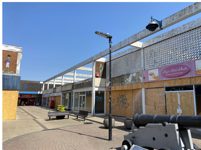
Figure 3 Shows the distinctive external concrete supports which are a feature of all four blocks, including Block B as shown. The photograph also shows the poor condition and vacancy of the ground floor retail units.
