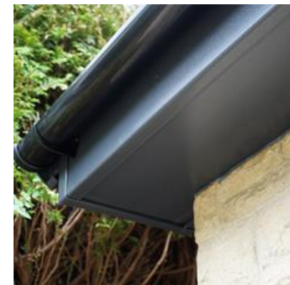
Anthracite Fascias and Soffits
