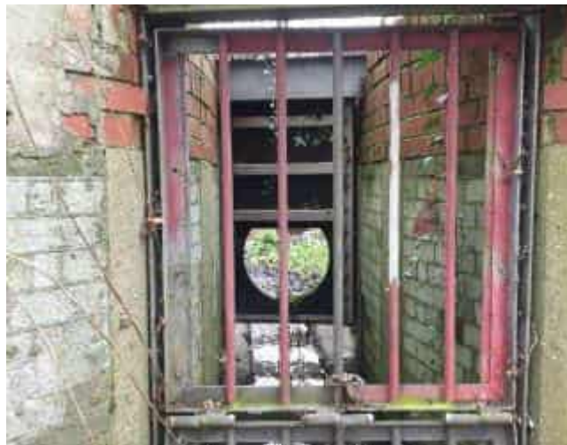
Figure 3: Penstock control structure downstream of Lavant Link Pipe
