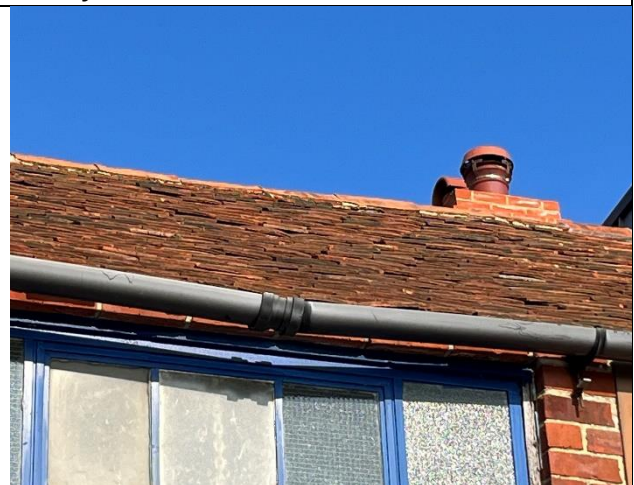
Photograph 4: Raised roof tiles on the two-storey roof.
