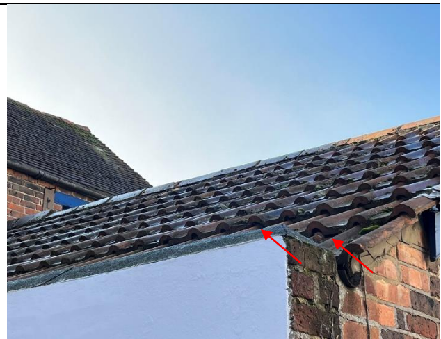
Photograph 2: Raised tiles on the single-storey roof.
