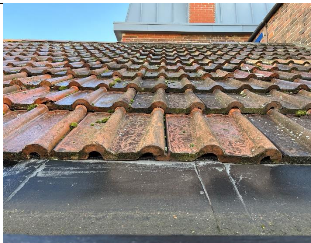
Photograph 3: Gaps within the bottom row of tiles on the single-storey roof.
