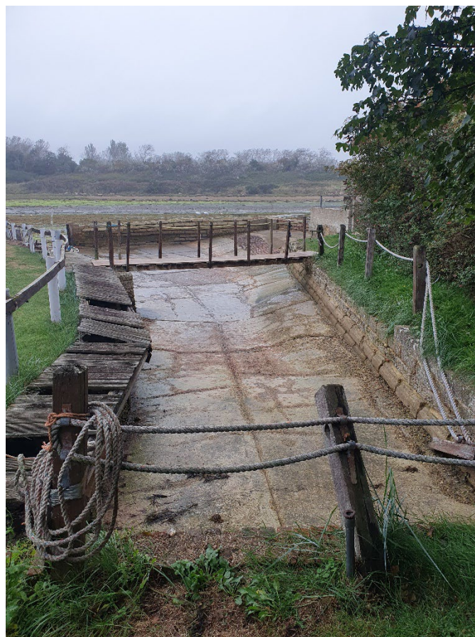
View looking north down dock. Note damaged wall on left and temporary bridge replacement.
