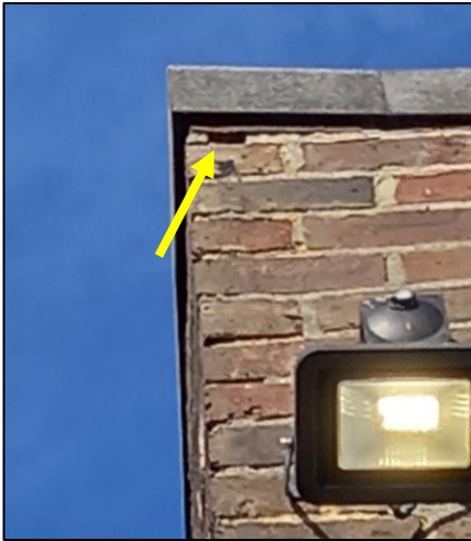
Photo 10 Section of missing mortar at south corner of building (feature 1)
