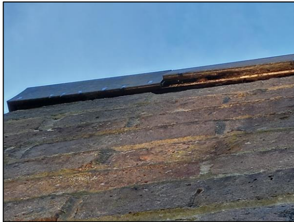
Photo 8 Overhanging lip of roofing felt over brick wall section
