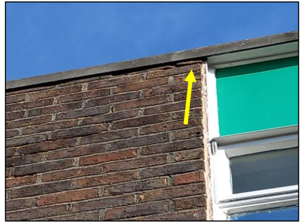
Photo 9 Missing mortar and small gap at top of panelling on SW elevation (feature 2)
