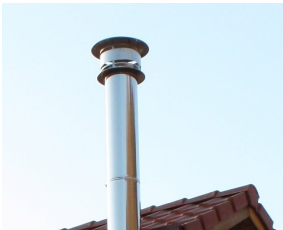
Stainless steel chimney flue
