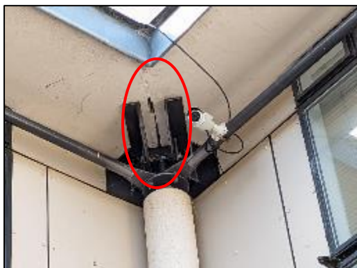
Figure 24: Crack within northwest corner of B1
