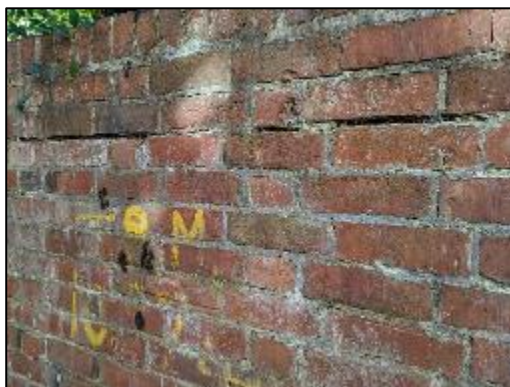
Figure 26: Gaps between bricks and mortar along southern site boundary
