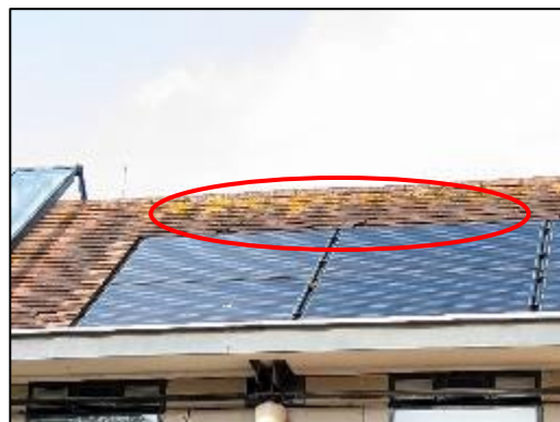
Figure 25: Missing tiles above solar panel on eastern elevation
