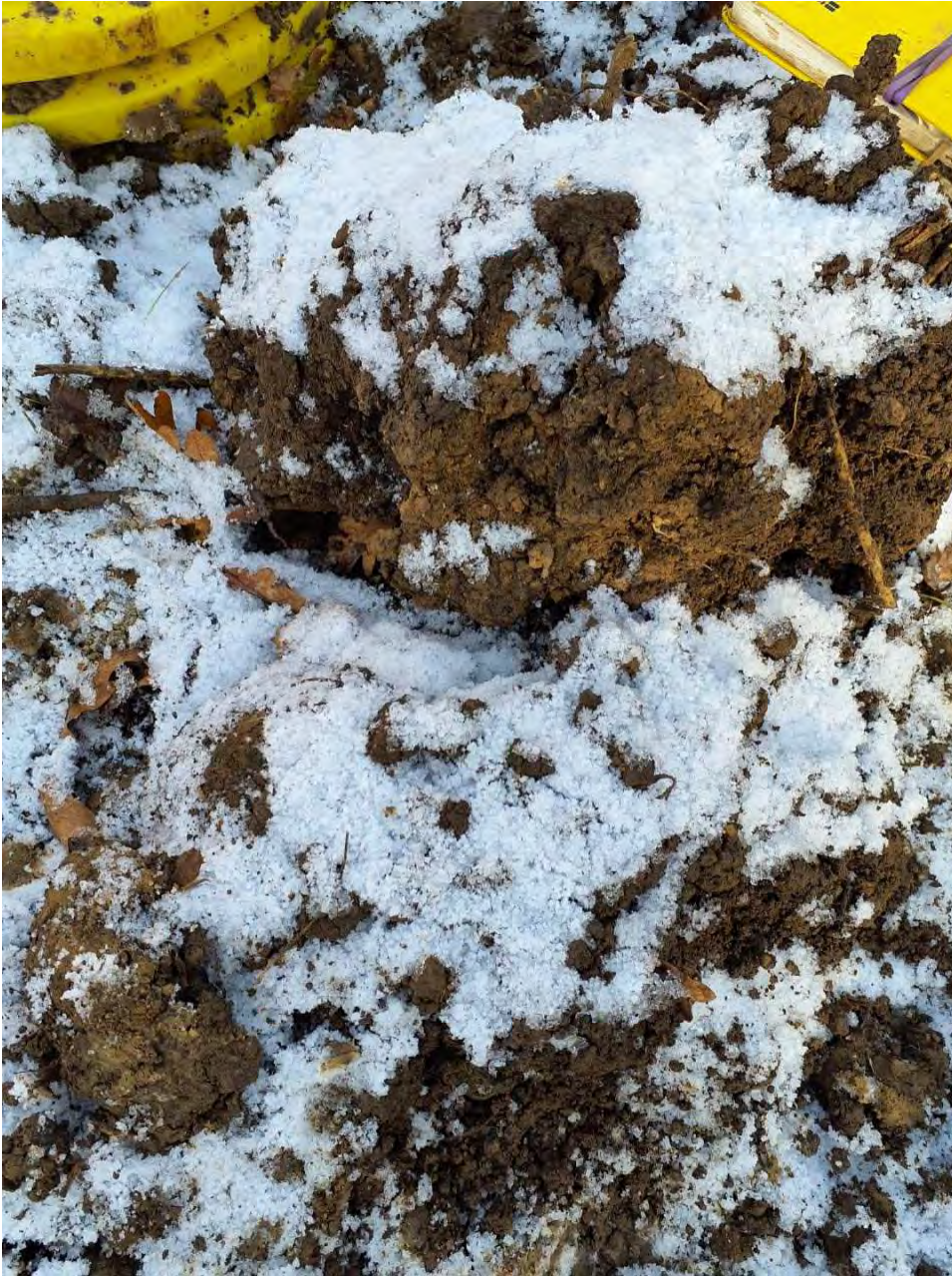
Photo of hole with tape in place
