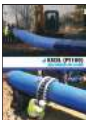
G0020 Large Diameter Pipe Systems
