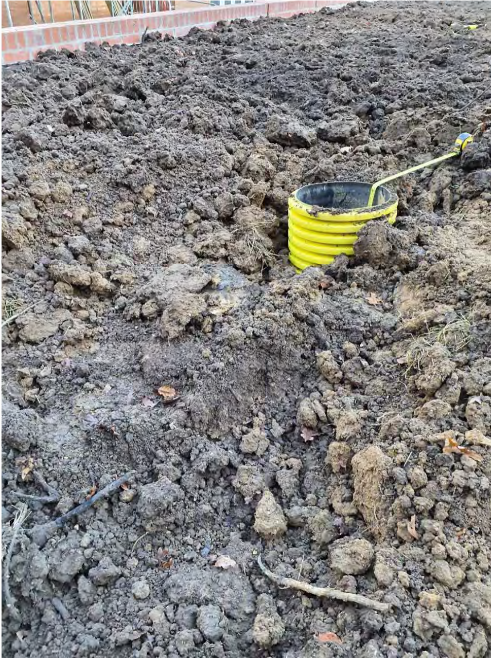
Photo of hole with tape in place
