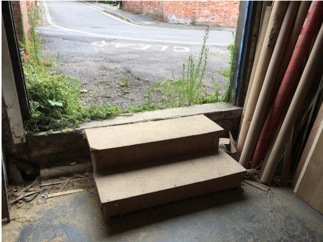
Non-DDA compliant access
