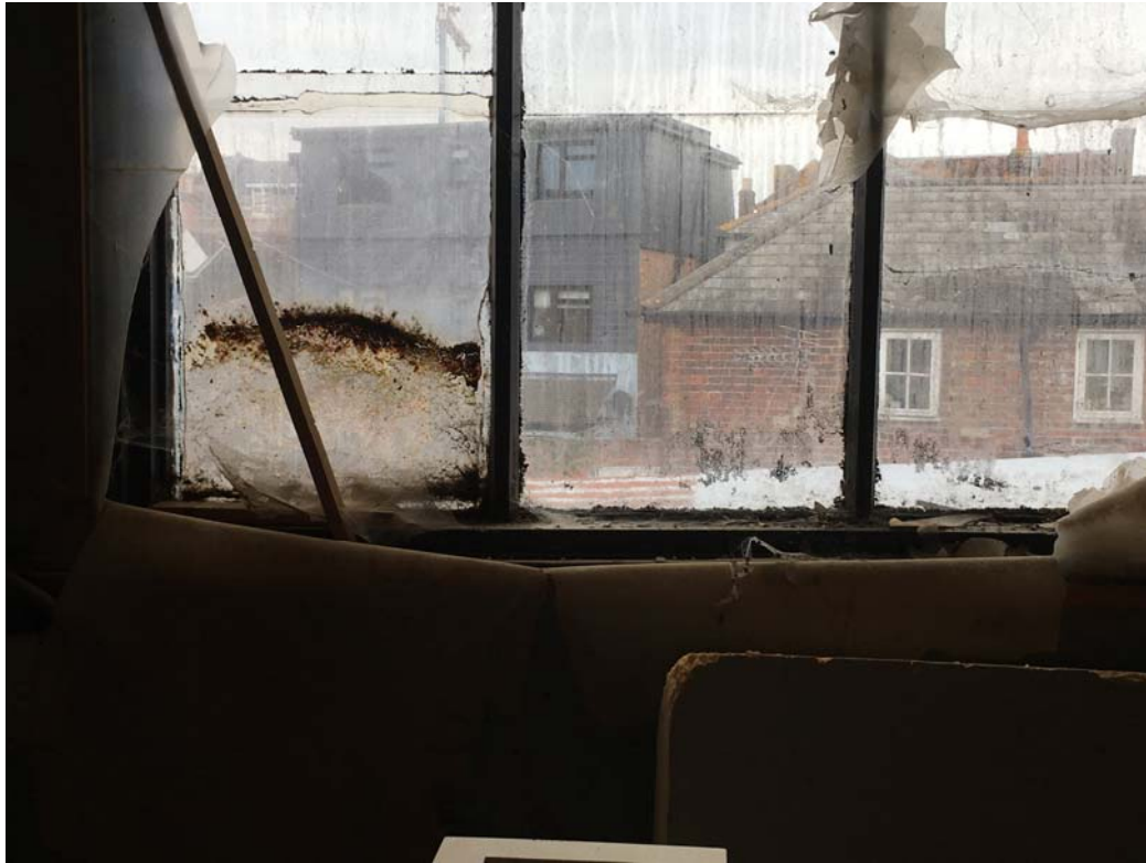
Failed Crittal windows
