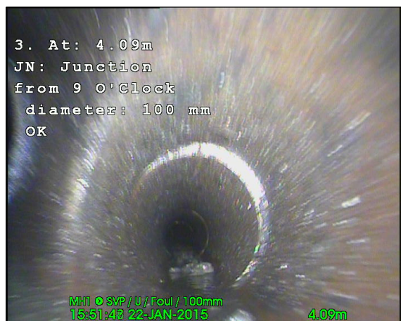
Photo: 150122_1551B-Survey.jpg 4.15m, Junction from 9 O'Clock diameter: 100 mm OK
