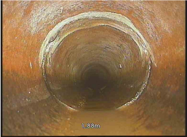
006.jpg, 00:00:21, 1.88 m Crack, circumferential at joint from 10 o'clock to 2 o'clock
