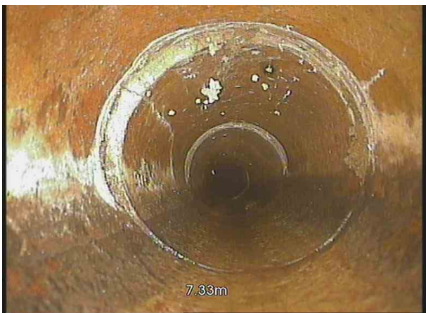
003.jpg, 00:01:05, 7.30 m Crack, circumferential at joint from 8 o'clock to 12 o'clock
