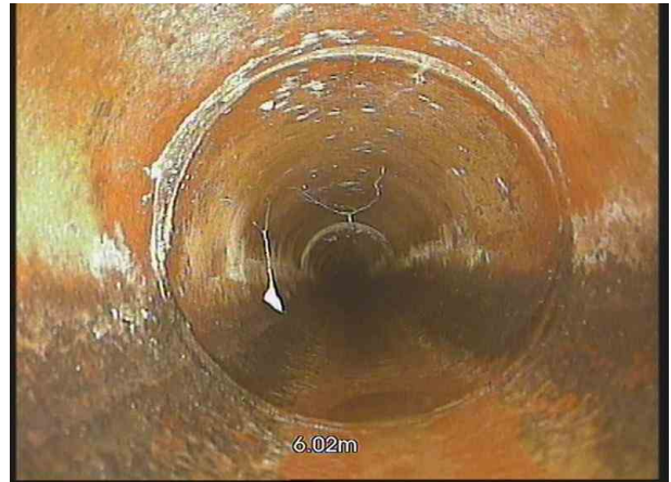
002.jpg, 00:00:50, 6.02 m Crack, circumferential at joint from 1 o'clock to 3 o'clock
