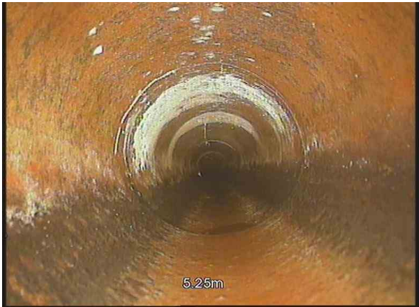
001.jpg, 00:00:41, 5.25 m Crack, circumferential at joint from 9 o'clock to 2 o'clock
