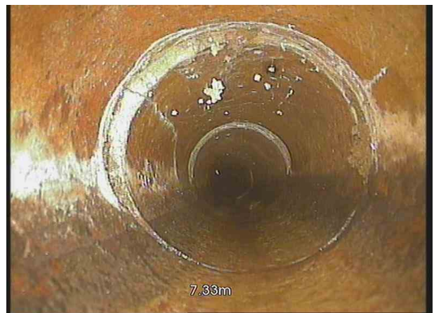
004.jpg, 00:01:07, 7.33 m Fracture, longitudinal at joint at 10 o'clock
