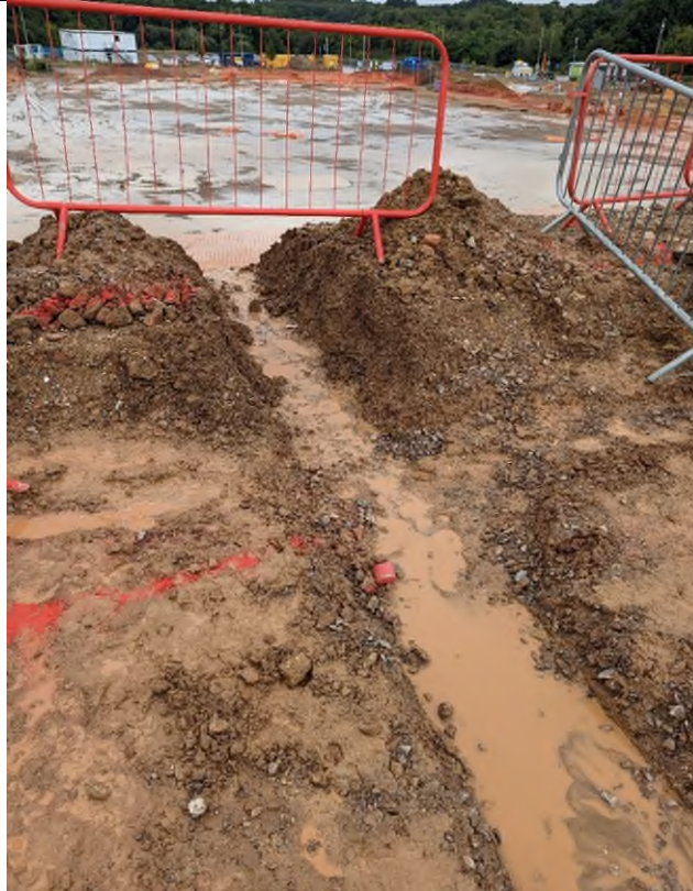
Photograph 10: Showing wet site conditions
