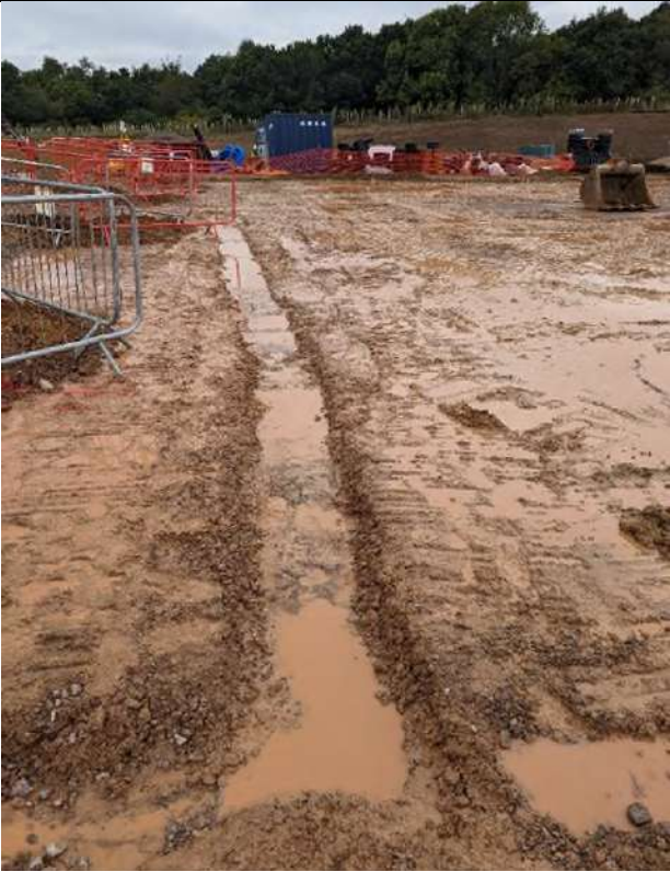
Photograph 10: Showing wet site conditions
