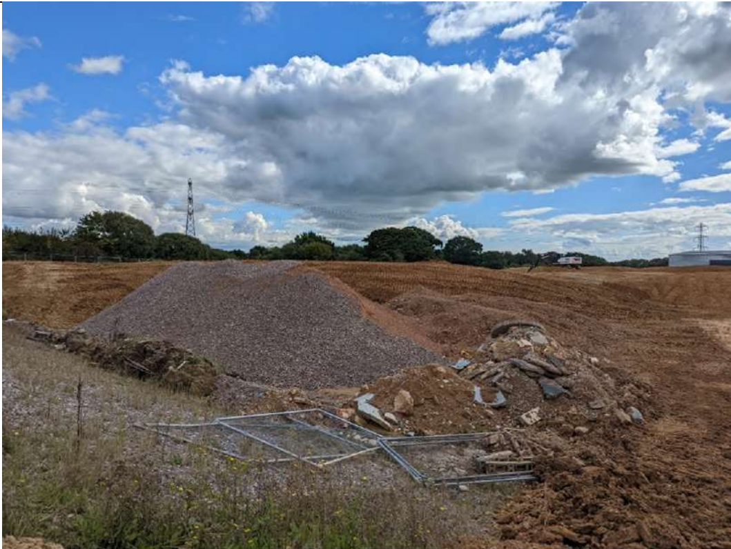
Photograph 10: Plot 400 showing some segregated stone and fly tipped material
