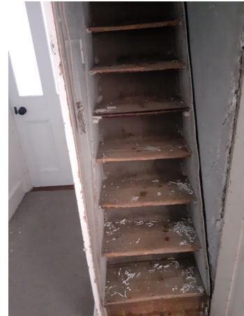
The existing dilapidated first-floor staircase.
