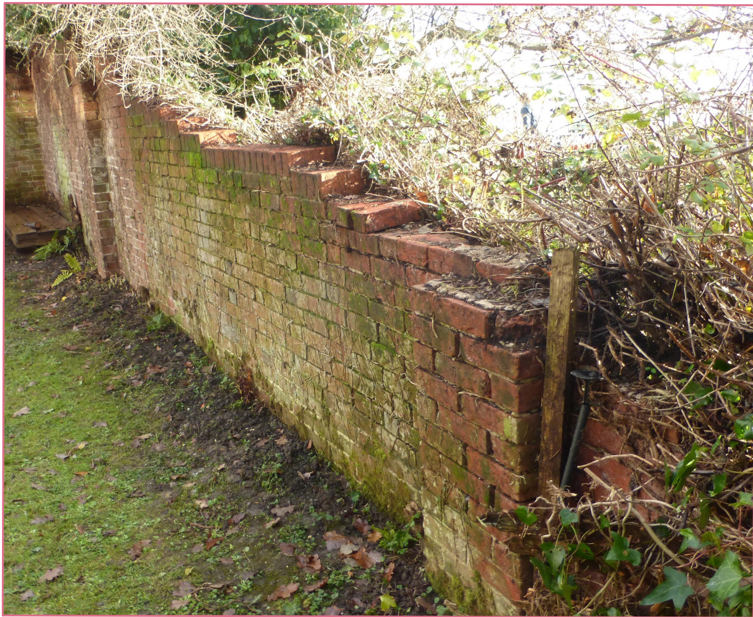
① — Stable Cottage garden wall, in need of vegetation clearance and stabilising
