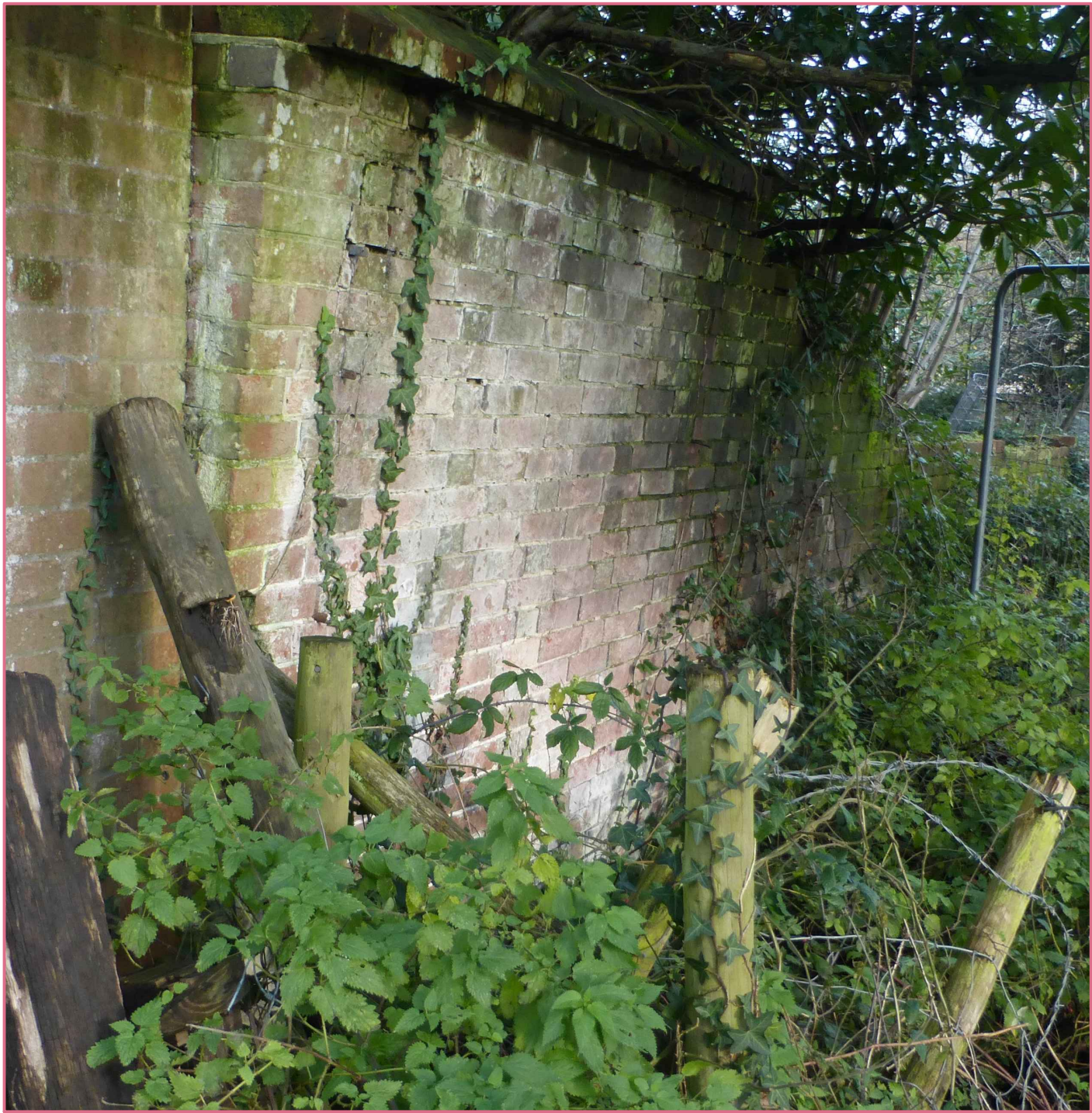
② — North west wall, in need of vegetation clearance, including fallen tree, and then the leaning wall will require raking shore to avoid future collapse.
