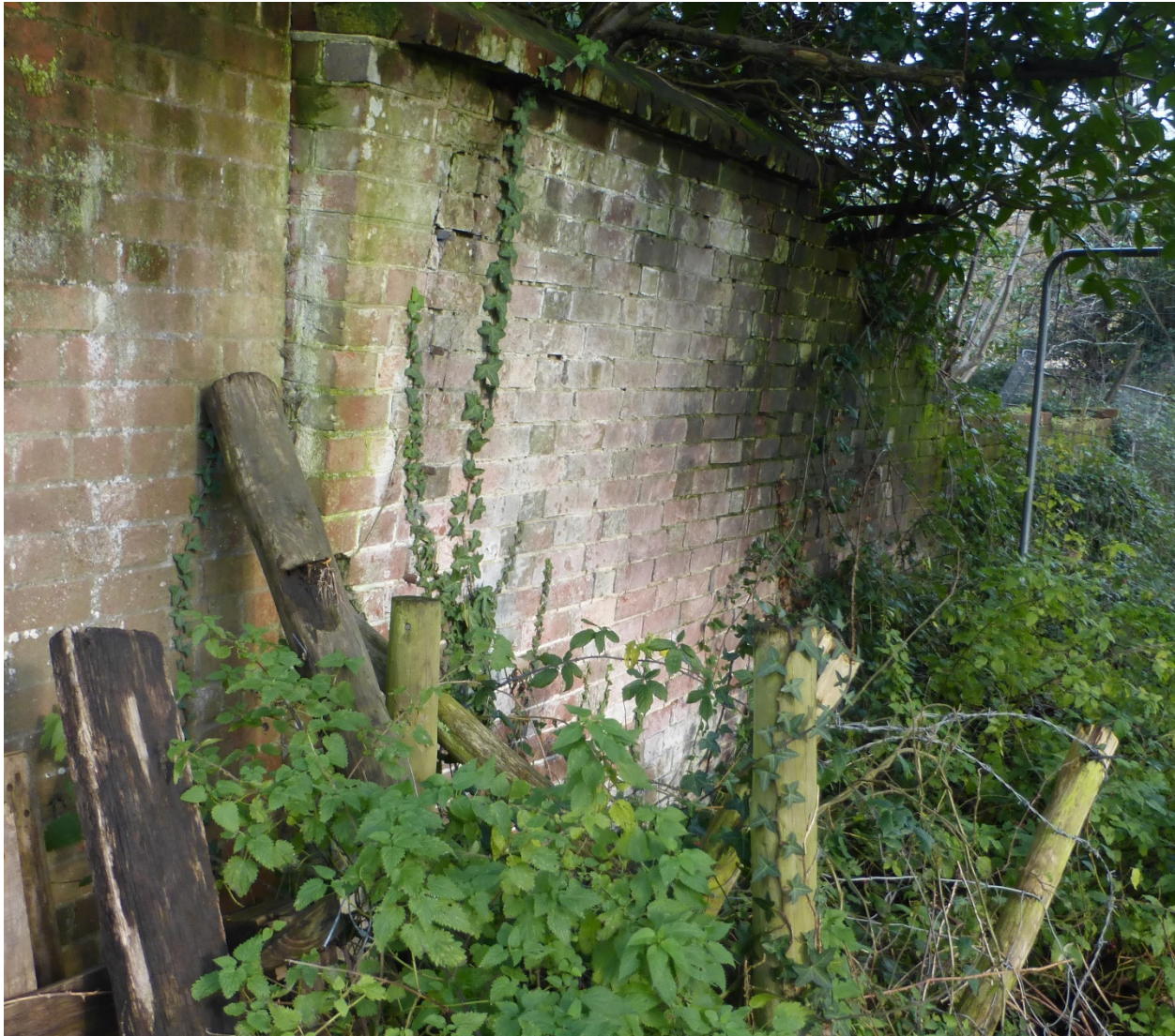
Fig 4: Image to show leaning wall
