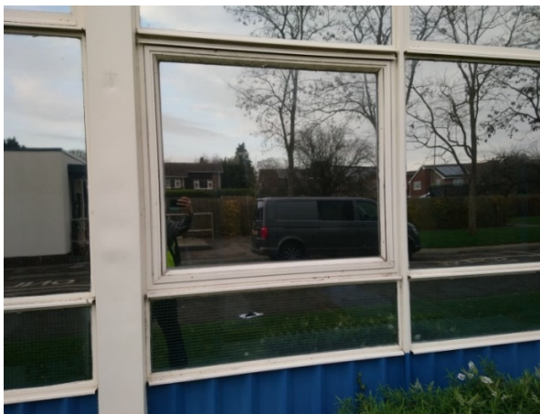
Fig 13: Closer image to show modern top hung window replacement - 3 Storey Block
