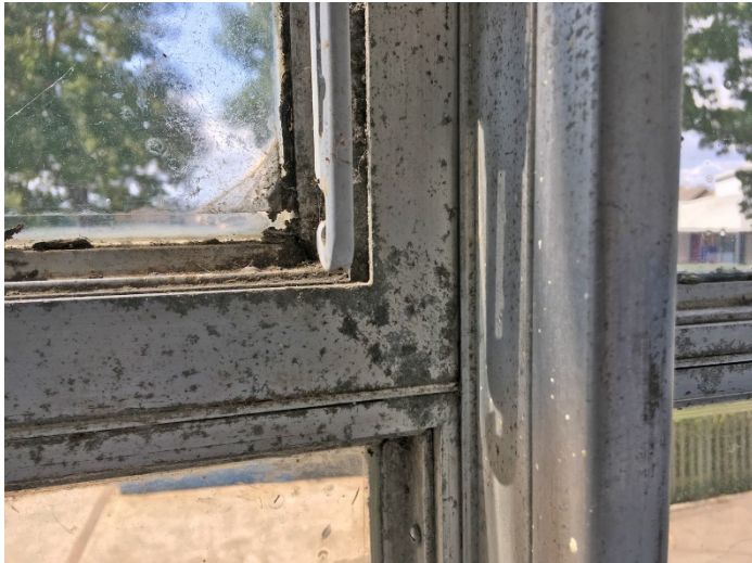
Fig 4: Modern replacement window, with problematic restrictor – 3 Storey Block
