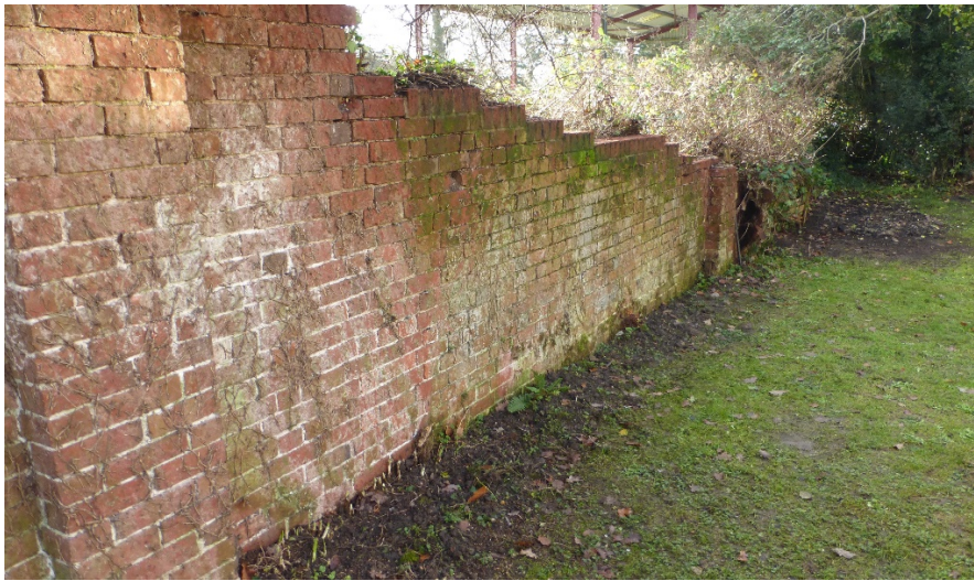
Fig 8: North wall viewed from within Stable Cottage garden, showing collapsed wall.
