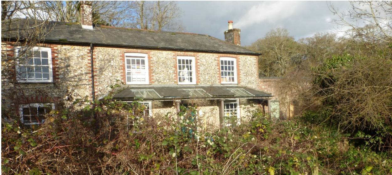
Fig 6: North wall historic collapse viewed from Storey Gardens
