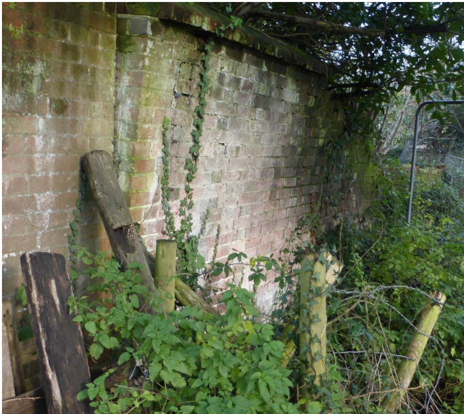
Fig 4: Image to show leaning wall
