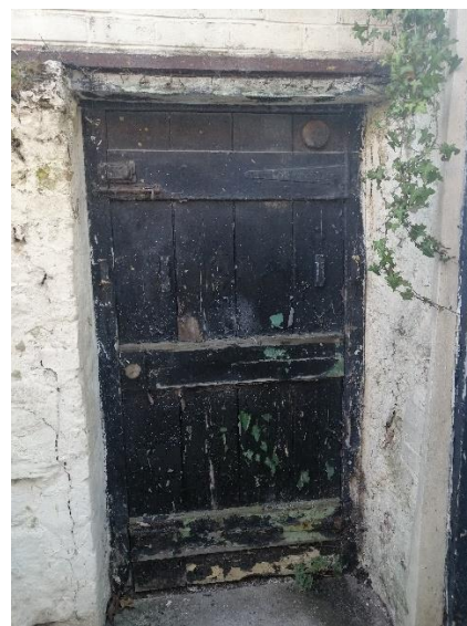
DG.10 to be fixed shut and refurbished
