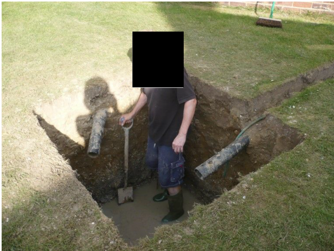
September 2012 – Soakaway in back garden showing water level in September
