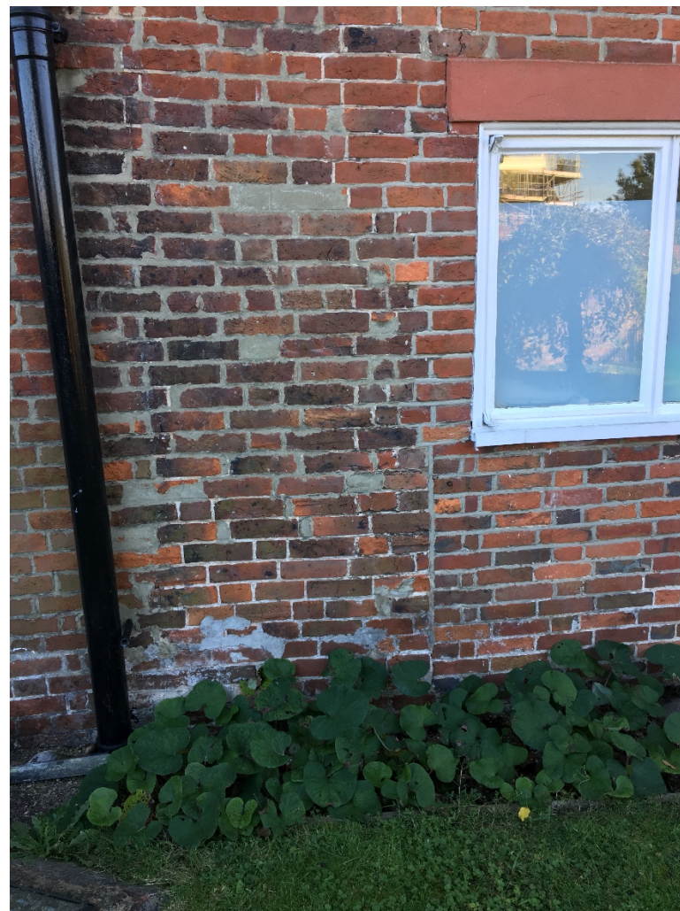
Plate 20: Break in brickwork at the centre of the north elevation.
