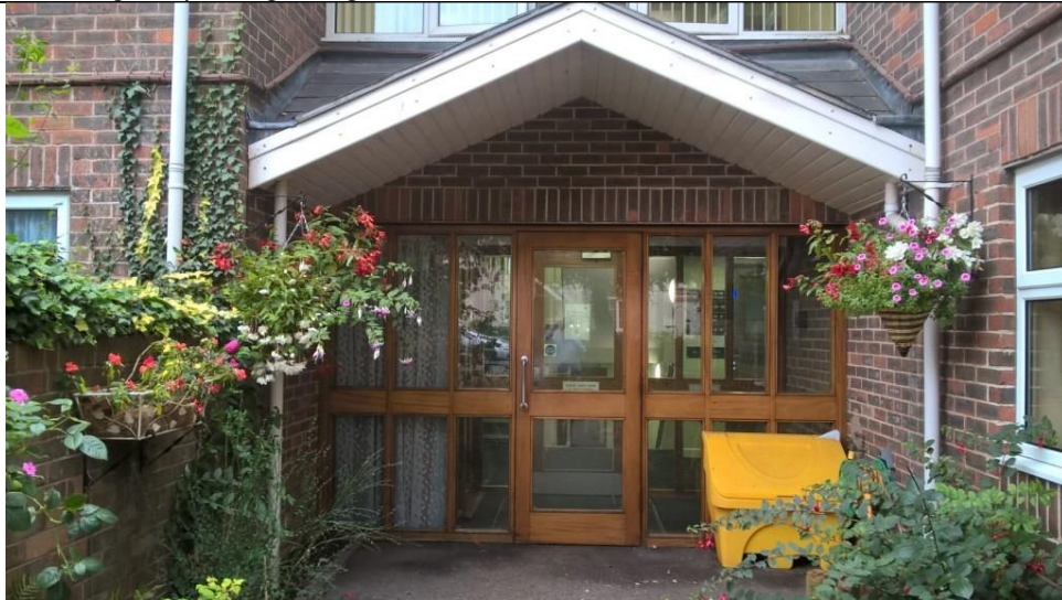
10. View of front entrance and dilapidated canopy. Proposal to replace with polycarbonate glazed dual pitched canopy to match style, with powder coated framework, and new grey powder coated aluminium automatic sliding entrance doorset.
