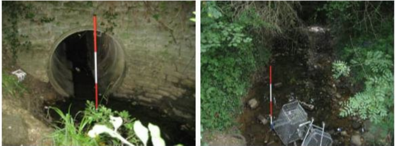
Photo 1: Major culvert & dumping in Riders Lane
