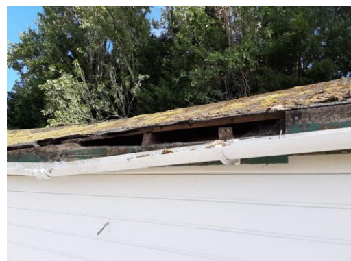
Plate 4.23: Damaged eave section on maintenance workshop building
