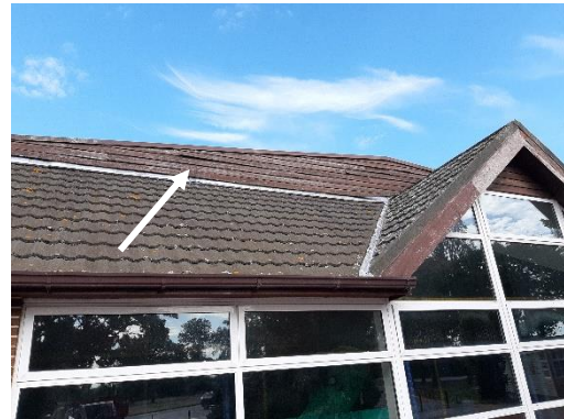
Plate 4.11: Damaged/lifted wooden boarding (arrowed)
