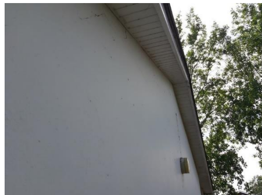
Plate 4.4: Tightly sealed soffitleave area accommodation chalets
