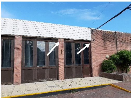
Plate 4.12: Gaps in brickwork (arrowed)
