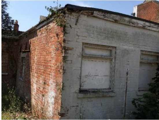
Photograph 3. Rotten flat roof and gaps beneath bargeboards.
