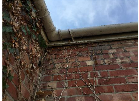
Photograph 4. Gaps under bargeboard of No. 9 East Street
