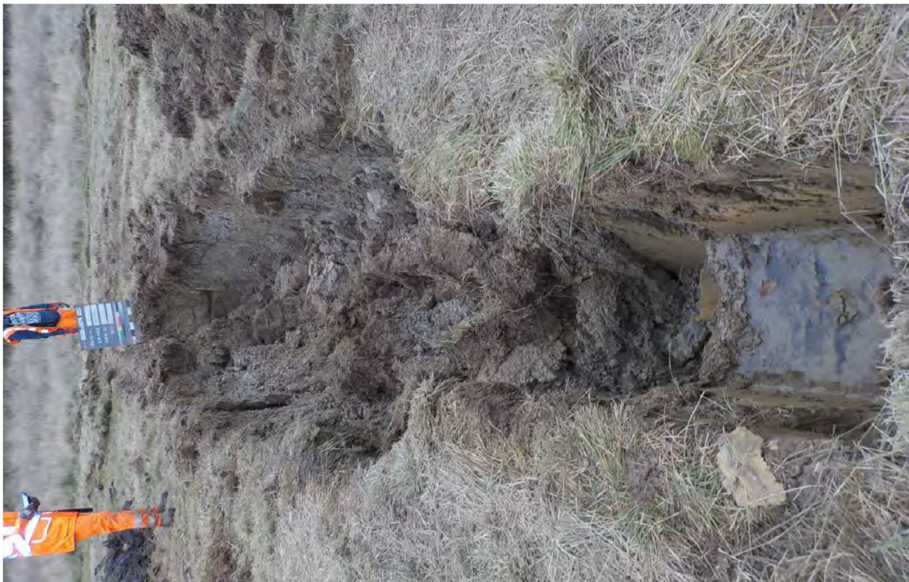
A9031-19 ATK-TPM-05 FACE D Collapse
