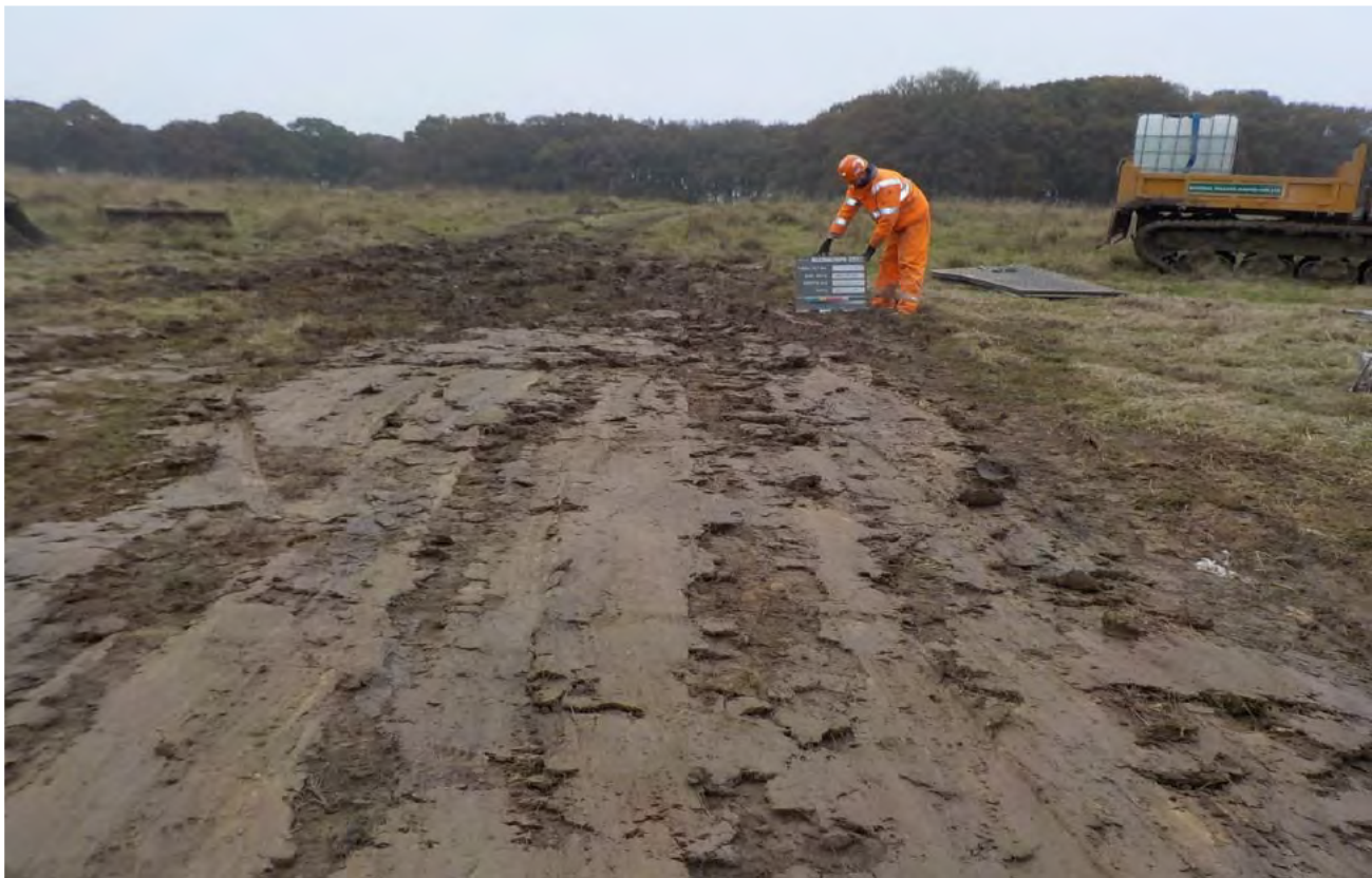
A9031-19 ATK-TPM-05 Post Condition
