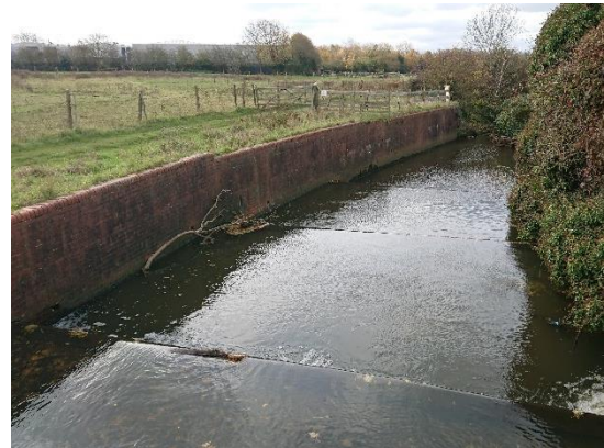
Photo 12: six-weir system on Hermitage Stream near to the NTL (approximate OSNGR SU 70648 06277).
