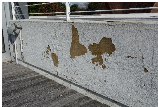
Significant problems in many areas of water penetration to substructure due to lack of damp proofing membranes and copings
