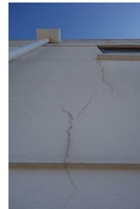
Significant cracking to finishes due to lack of movement joints in large areas of cementitious render and subsequent building movement
