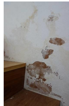
A number of internal areas of damp where the original cavity is failing and lack of DPC or failing DPC – poor ventilation further exacerbates many of these areas
