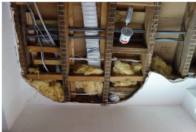
Large areas of wall roof and floors with no insulation and would require a major rebuild to accommodate
