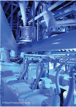
K Rend Production Facility
