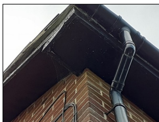
Figure 8 – damage to the south eastern corner of the eaves
