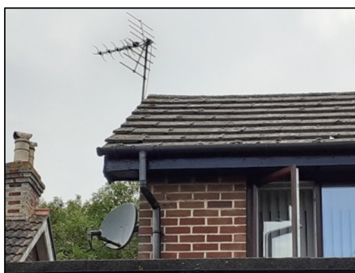
Figure 7 – Lifted roof tile at the southern end of the eastern roof face
