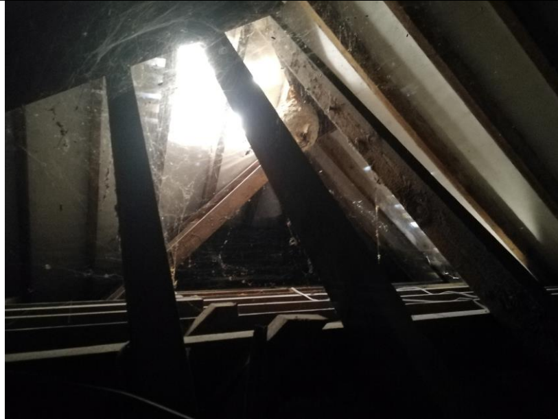
Photograph 15: View of dense cobwebs in roof void and hole in roof from the vandalism seen in photograph 2. Lining present behind tiles.
