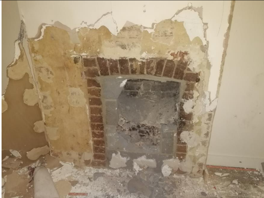
Photograph 11: View of vandalised chimney. All chimneys searched for evidence of bats on floor and up the stack
