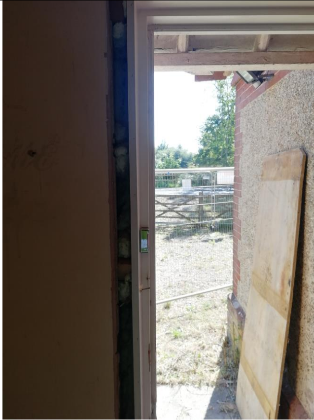
Photograph 13: View of missing door framing providing crevices. All such features could be fully examined for evidence of bats at time of the survey
