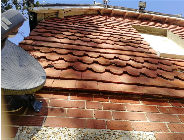
Photograph 3: Hanging tiles with gaps behind on the eastern elevation of The Gable
