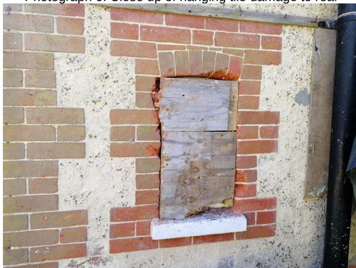
Photograph 7: Examples of windows blocked up. Smashed glass behind.
