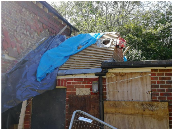
Photograph 5: Pitched roof extension with all tiles missing and hole in roof
