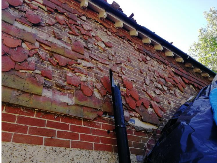
Photograph 6: Close up of hanging tile damage to rear
