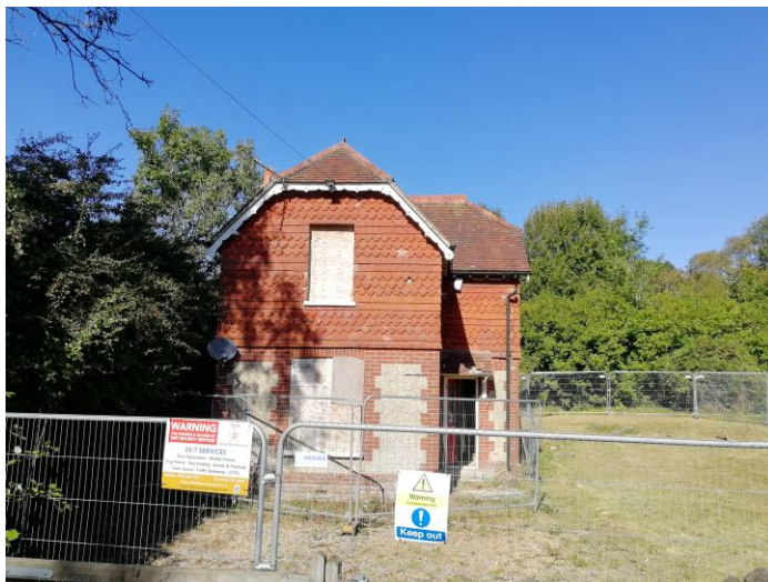
Photograph 1: The front of The Gable property, with a couple of missing hanging tiles present
