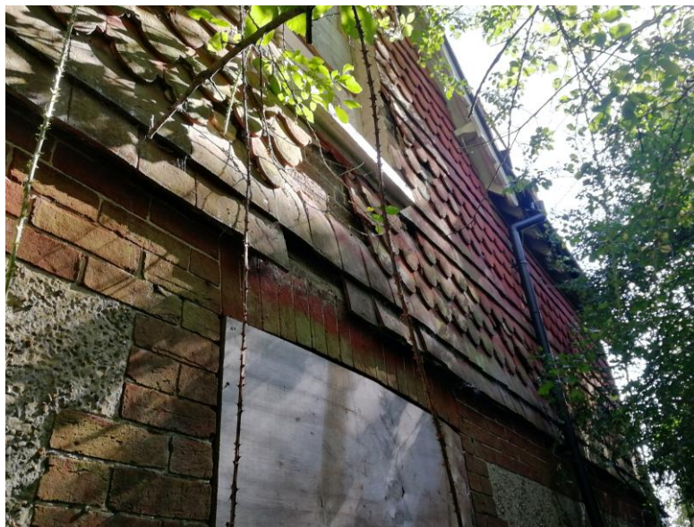
Photograph 8: View of missing hanging tiles on western elevation
