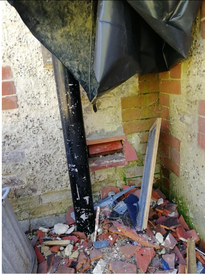
Photograph 9: View of missing vent with brick jammed in it. Gap visible from interior and no evidence of bats
