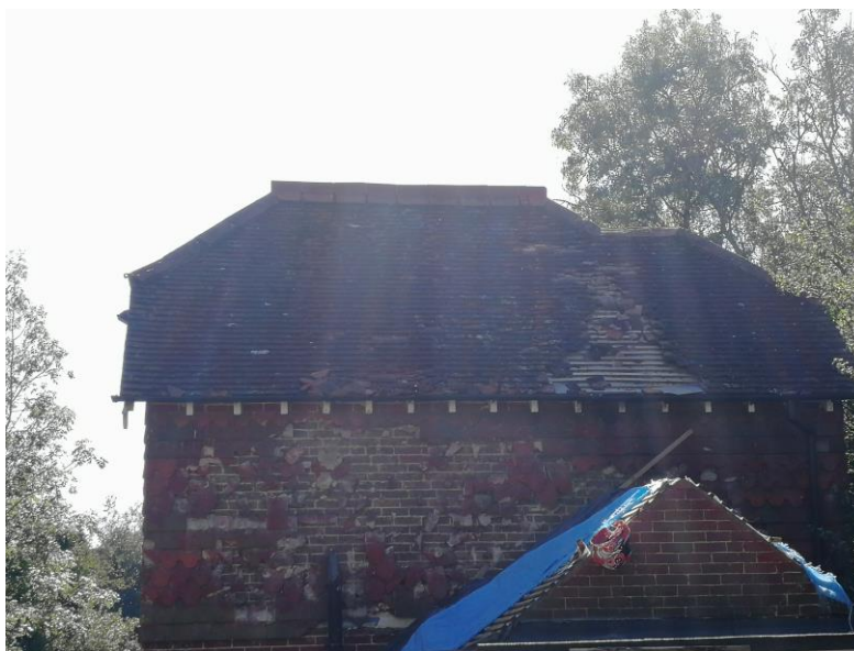
Photograph 2: View of the rear of The Gable with extensive missing roof and hanging tiles
