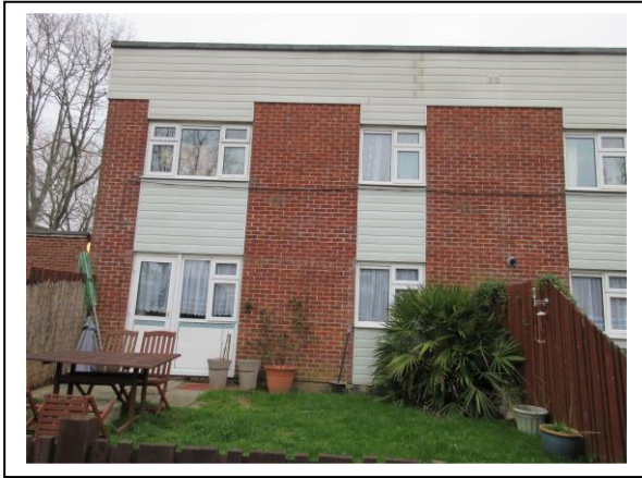
Fig. 1 - PVC ship lap cladding to be replaced with fibre cement cladding boards
