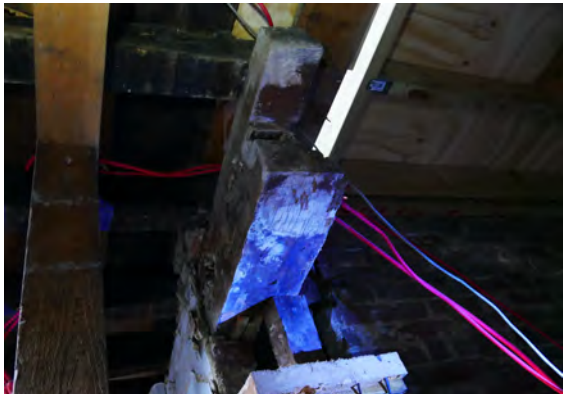
24. Disengaged side girt of the original 3-bay timber frame. Intruded into with formation of doors to G11 & G12 as well as west extension.
