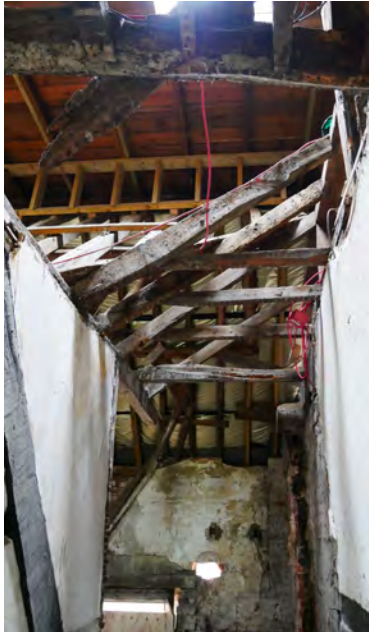
87. Fire damage to timbers that have been reused. Rafters spanning FF14/17 raising height along with north cross wing.
