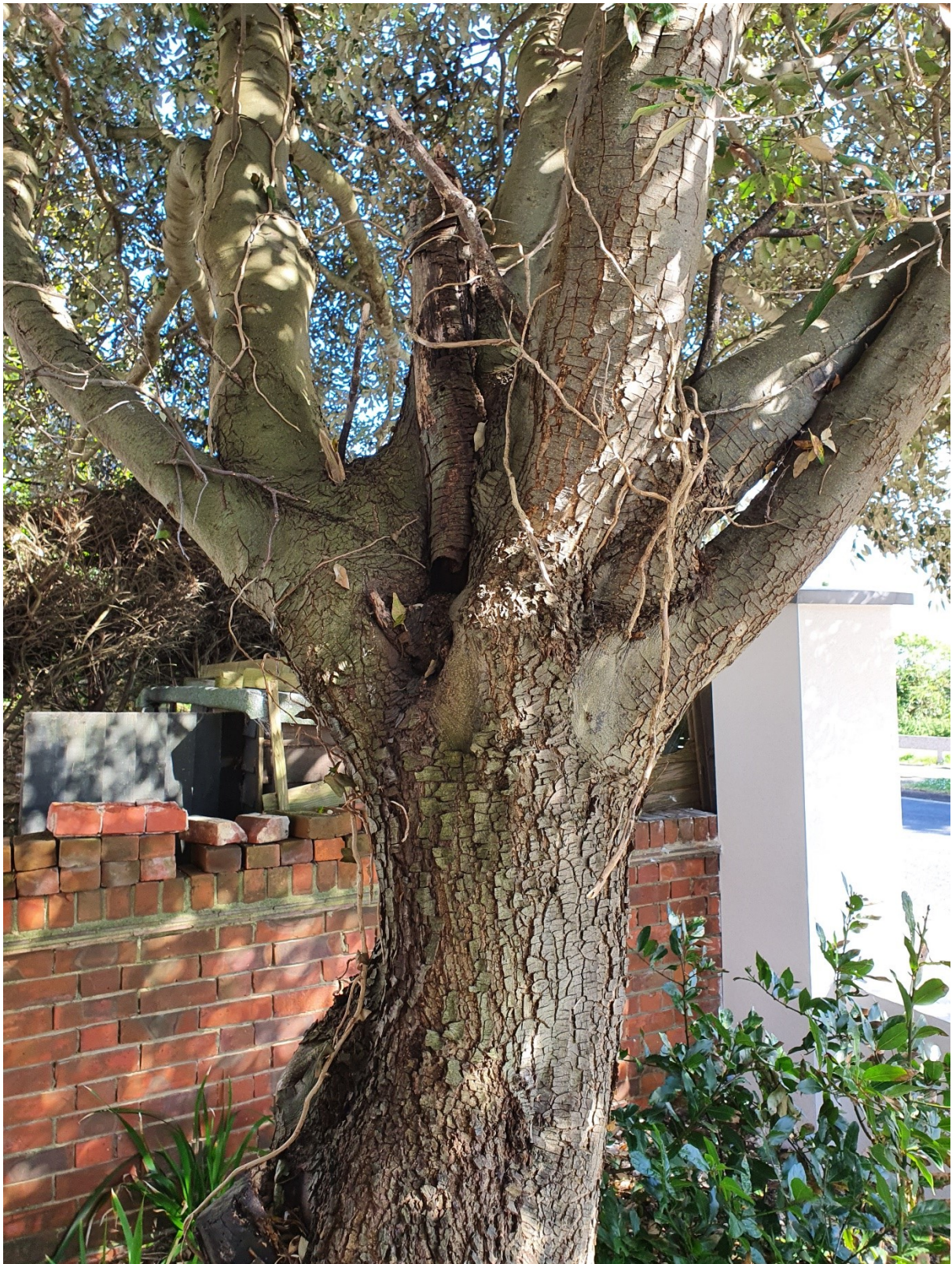
Figure main unions poor attachments
